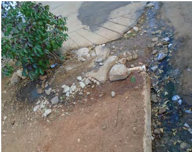
Photo 5.3-14 - open-air sewage discharge at the headquarters of Capitão Gervásio Oliveira (02/11/2016).
