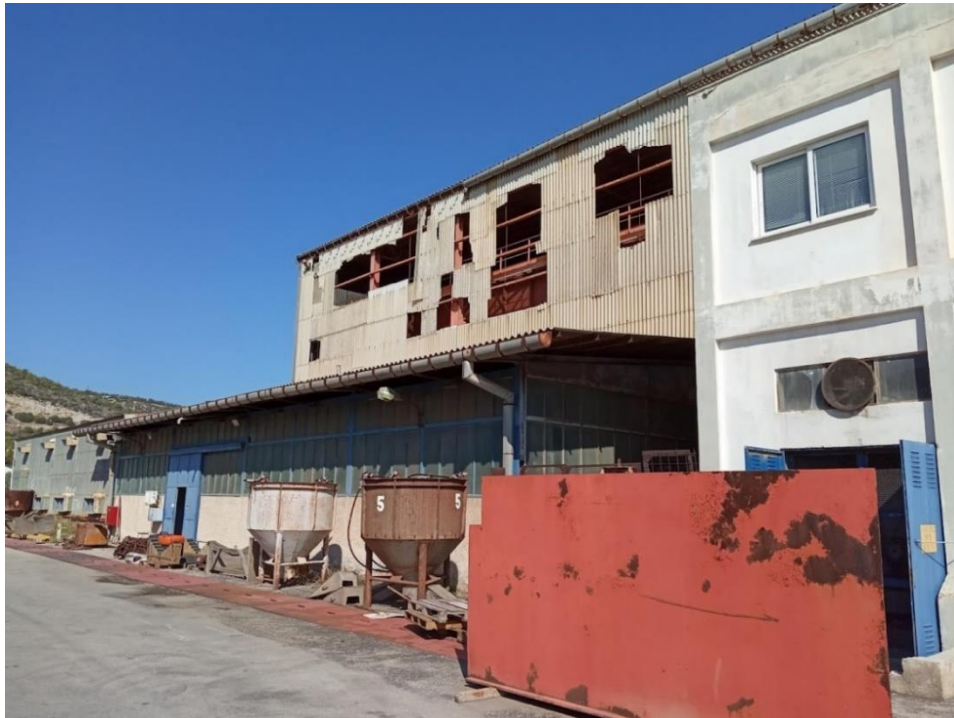
Figure 3.23: Asbestos present in damaged wall cladding
