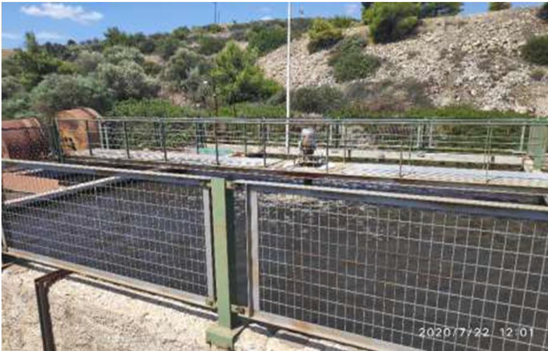
Figure 3.12: View of the Biological Treatment Unit
