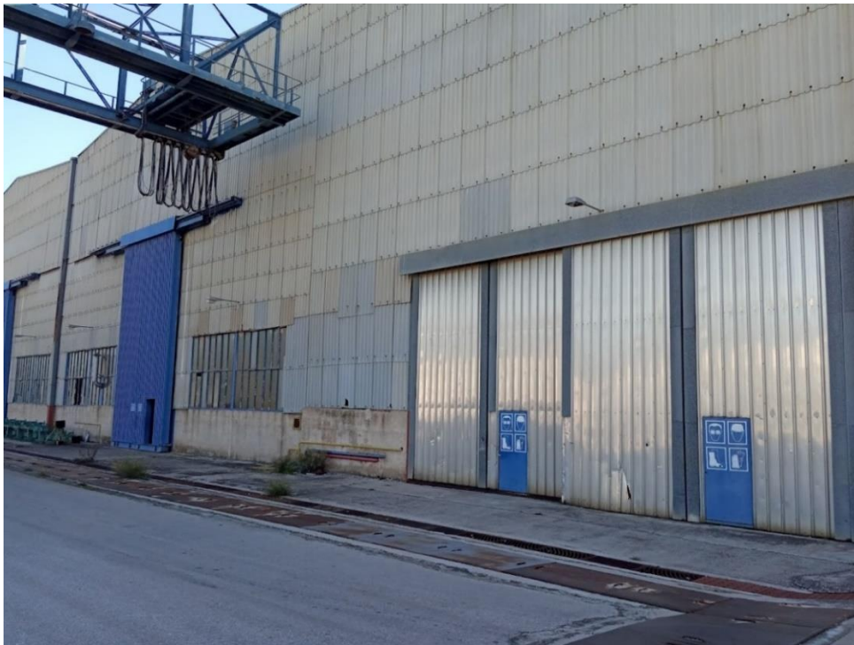
Figure 3.24: Asbestos present in wall cladding (2)
