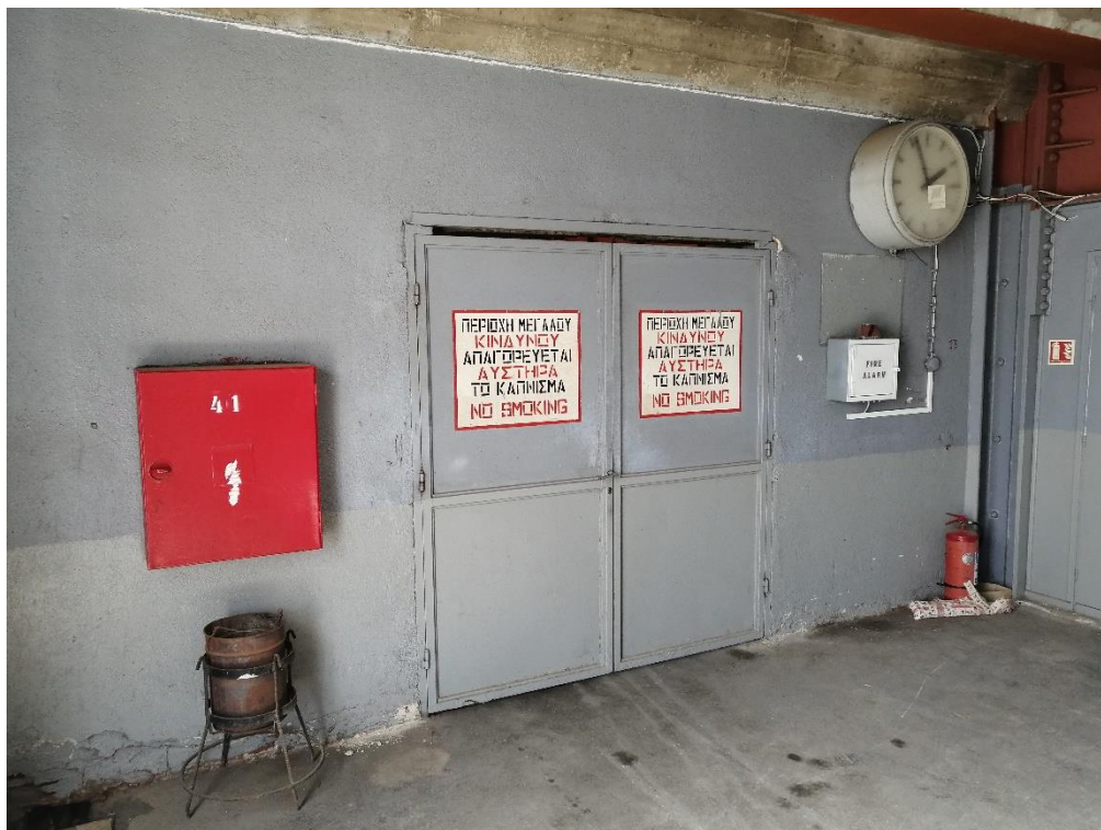
Figure 3.27: Safety signs in the entrance of Chemicals Warehouse
