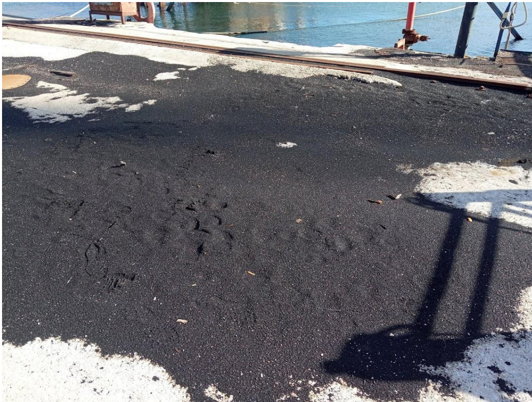
Figure 6.8: Blast sand found on pier
