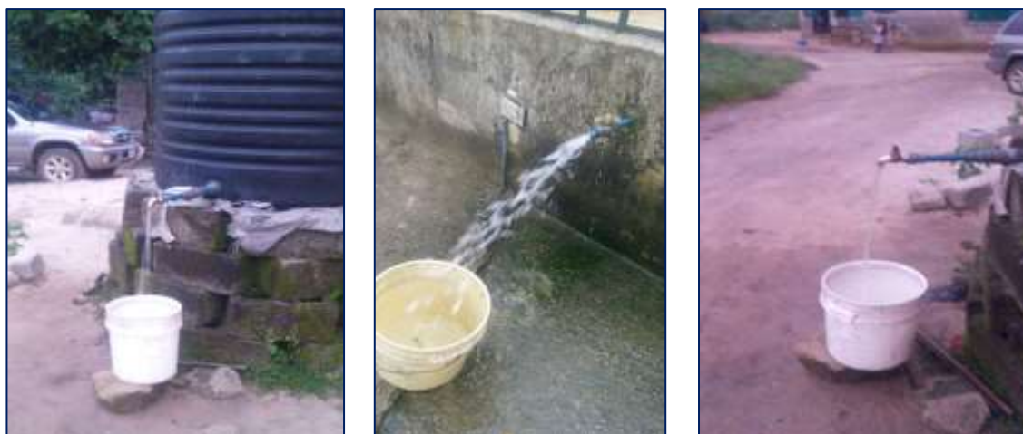
Plate 4.11.5: Water taps at Agbonchia
