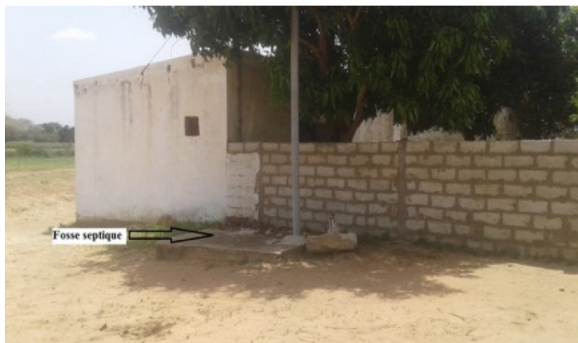
Photo 12 : Wastewater management- septic tank of ASUFOR of Malicounda Wolof
