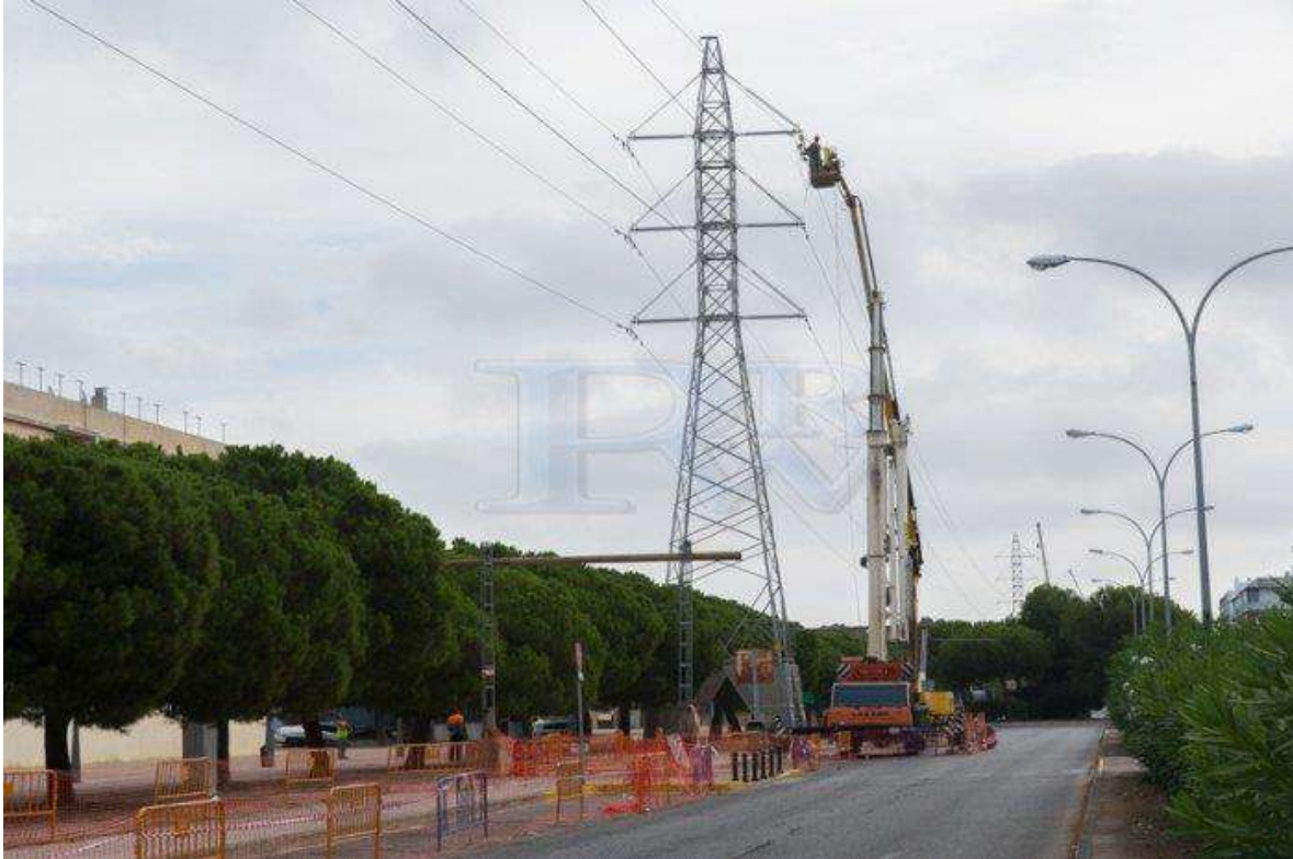
Illustration 7: SUITABLE SIZE CRANES TO THE AREA OF ACCESS ARE USED IN THE ACTIVITY OF LAYING AND TENSIONING.
