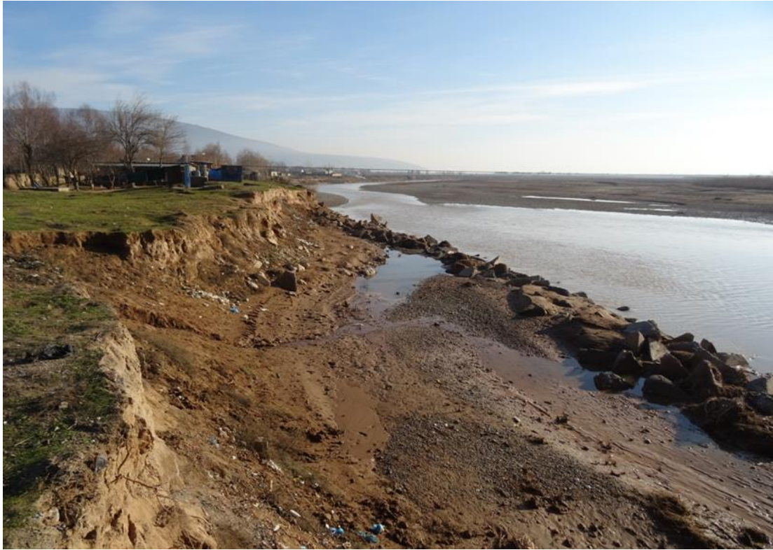
Photo 12 Damaged left bank of Kizilsu river
