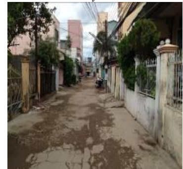
Degraded concrete alley
