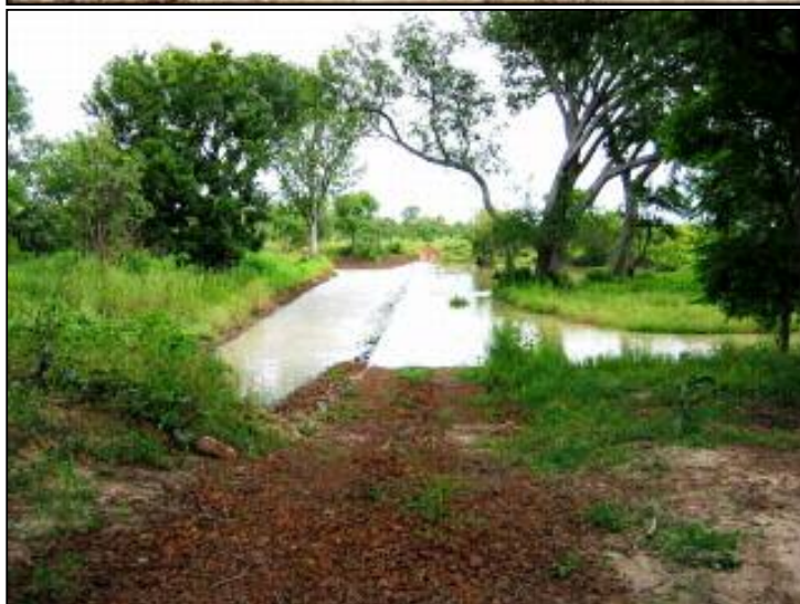
Figure 7: A shallow flow at the Naguio Spillway Dike, where the depth of the flow can be over 1 m in height (for reasons of cost-effectiveness the length of the spillway was designed to permit passage during the most, but not all, of the rainy season, as passage immediately after a heavy rain is not essential at this crossing)
