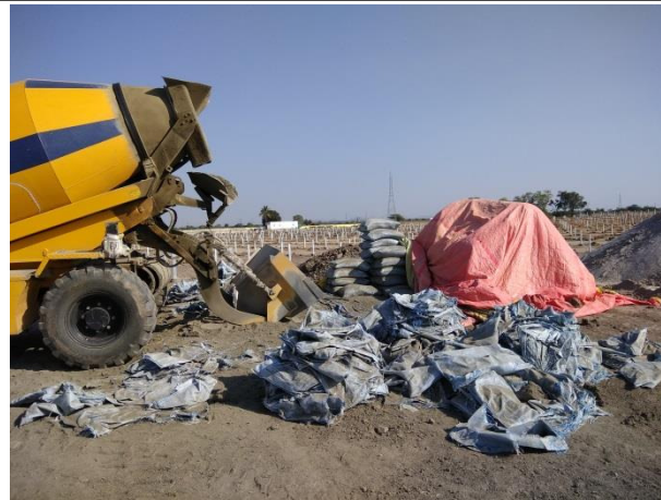
Photo 11: Empty cement packet kept at project site
