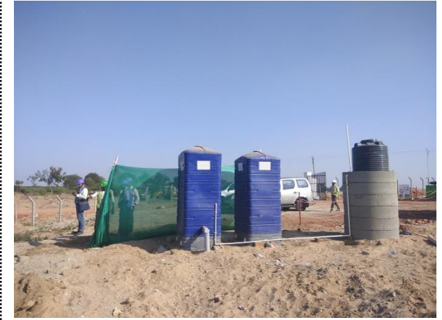
Photo 3: Sanitation facility at Balledupalle site
