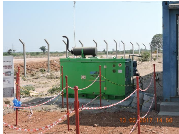
Photo 4: DG set at Balledupalle site
