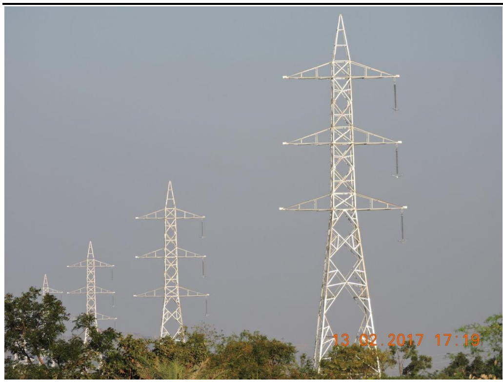
Figure 2.6 220 kV Transmission Line
