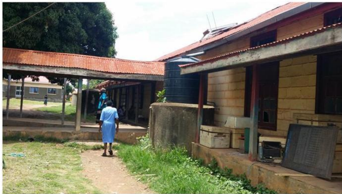
Femalepatients' Ward with faulty solar system
