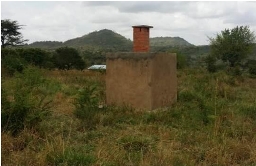
Plate 1: This masonry kiln “incinerator” at Kamion Health Center II was poorly designed and its construction was never completed.
