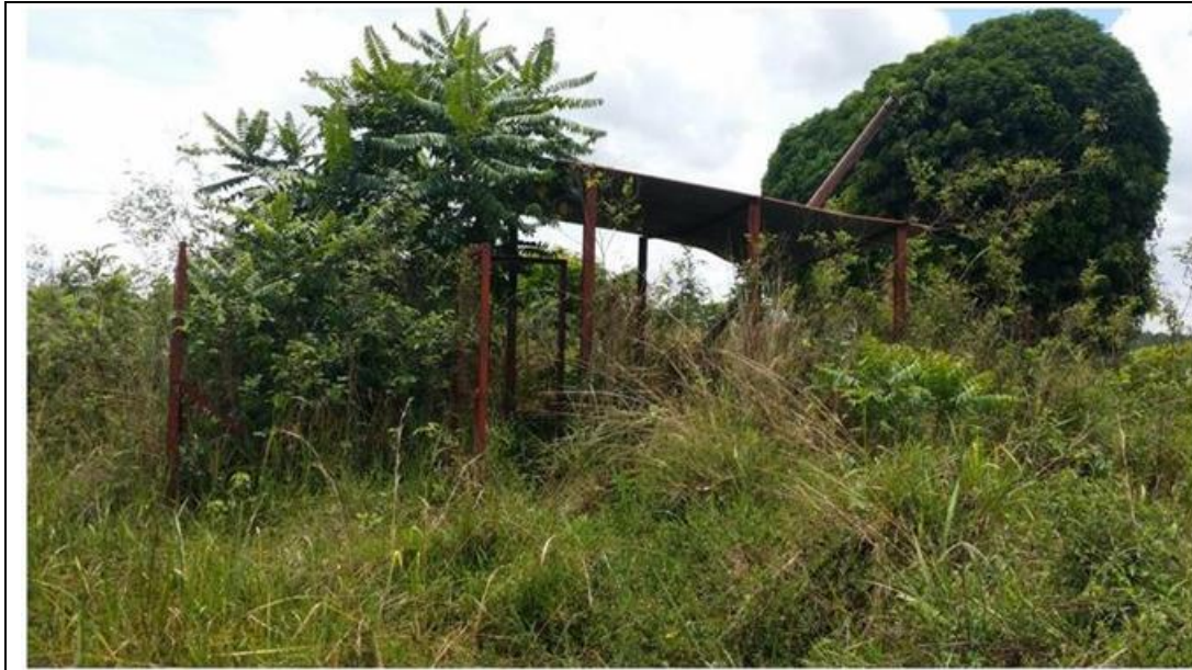
An derelict incinerator that was never used due to poor design
