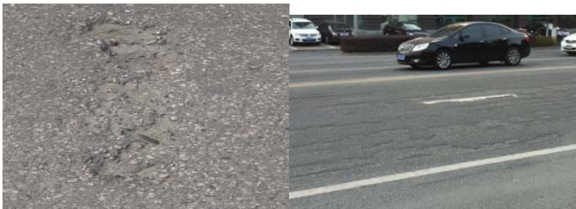
Status of Damaged Pavement of Tianan Lu
