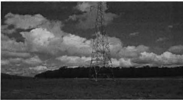
Figure 9-12: The T/L Crosses Sodd – Sauala 132 kv Transmission Line between Bend 5 & 6
