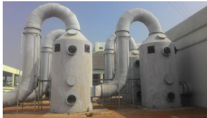
Picture 7.1. Odour Treatment Tower at Thu Dau Mot WWTP
