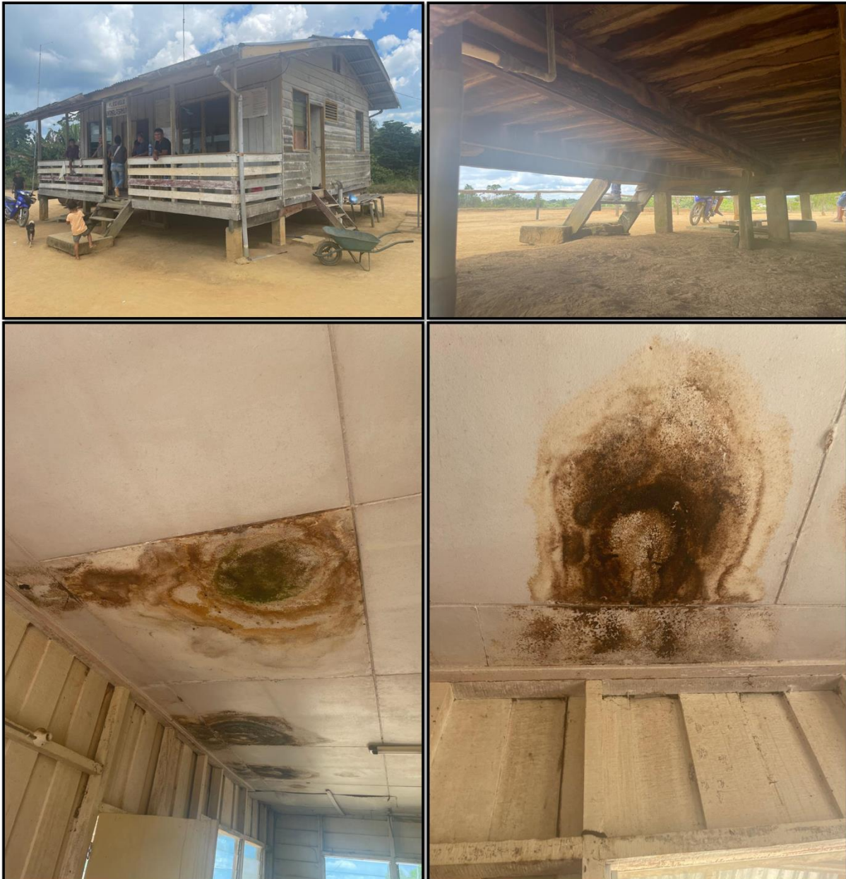
Figure 48. Station building signs of deterioration. Source: PlanEHS, 2024.
