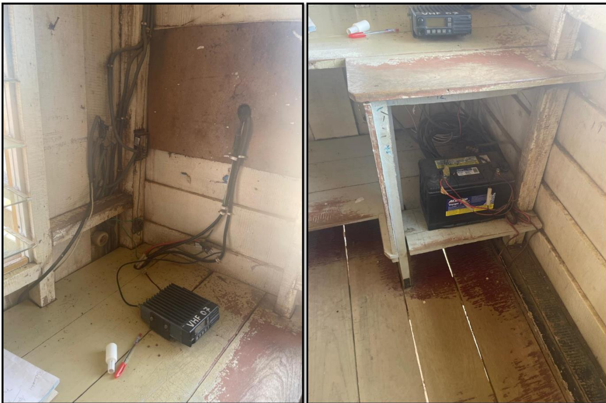
Figure 50. Non operational communication system in Station Building. Source: PlanEHS, 2024.
