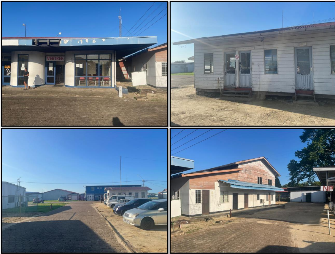
Figure 56. Signs of deterioration in Zorg en Hoop Airport buildings. Source: PlanEHS, 2024.
