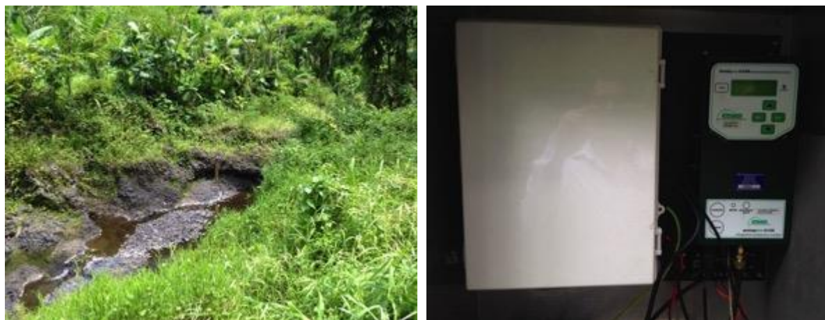
Figure 3 Hydrological monitoring station in Samoa
