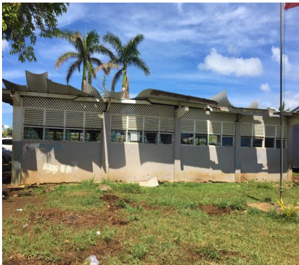
Figure 7 TC Gita: Major Damage to 8 classrooms at Vaini Government Primary School
