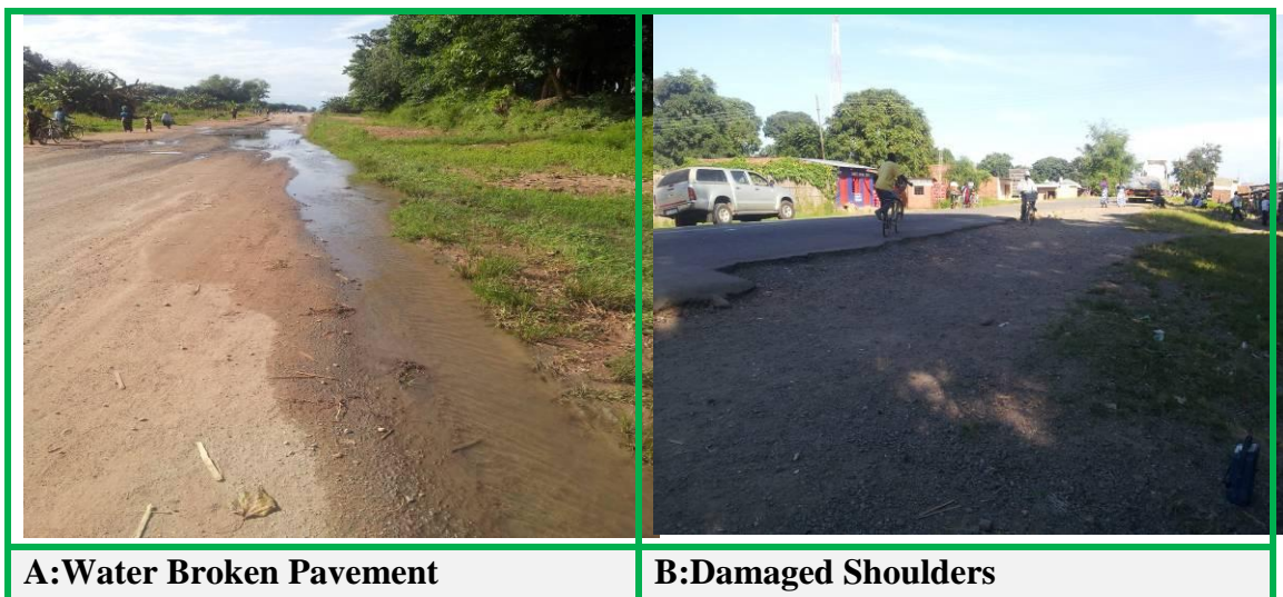
Figure 2: Some sections of the road which are in bad shape
