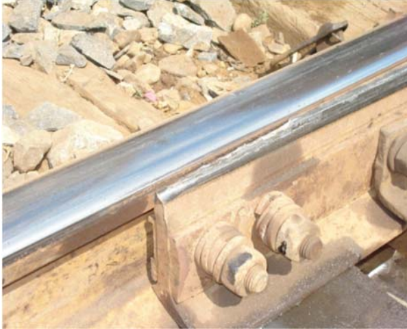
Damaged point blade
