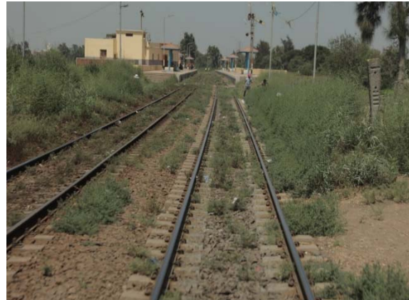
Contaminated ballast with vegetation
