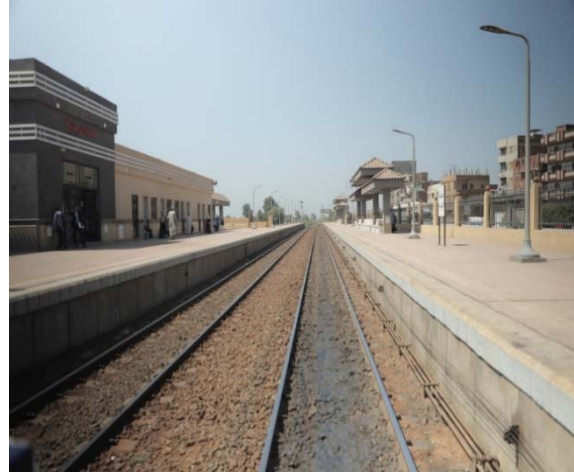
Contaminated ballast with debris, dust and oils at a station
