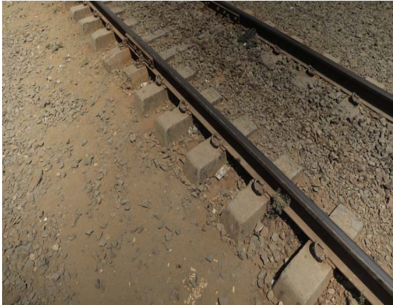
Lack of ballast / contaminated ballast
