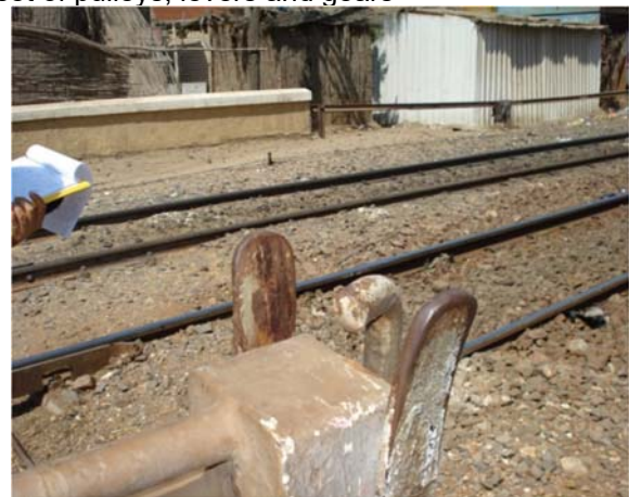
Detail of blocking system of mechanical Local Control Panel barrier
