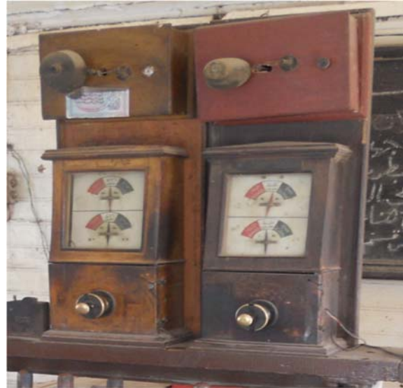
Block n° 6 is electrically controlled from Tanta station
