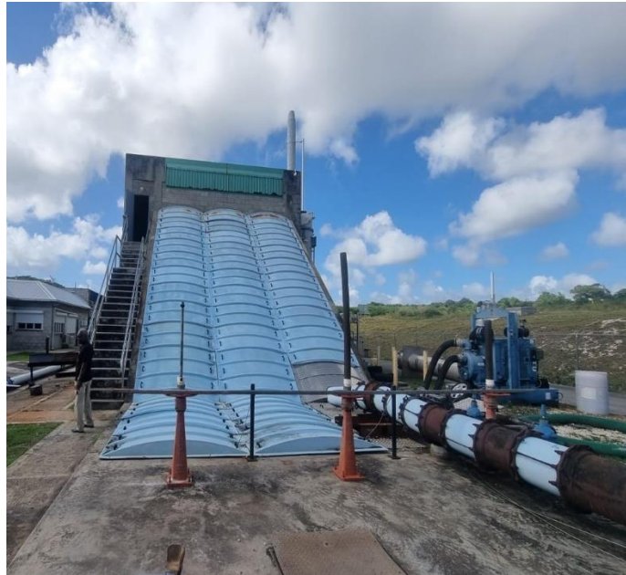
Figure 5-10: Headworks at the Existing SCSTP
