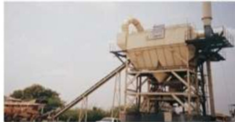
Hot Mix Plant
