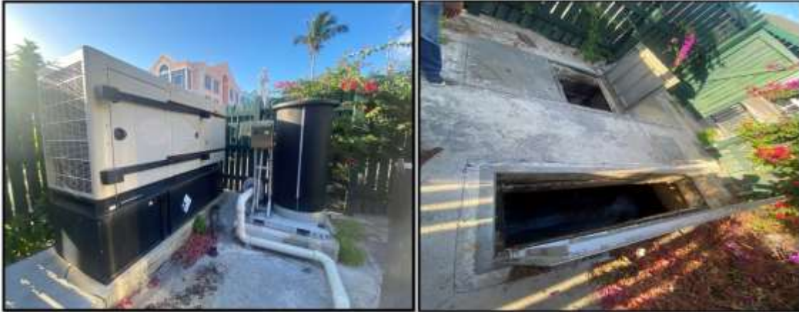
Figure 141. Rawson Square Lift Station: (a) power generator and Chlorination Dosing Machine; (b) well chambers. Source: PlanEHS, 2024.
