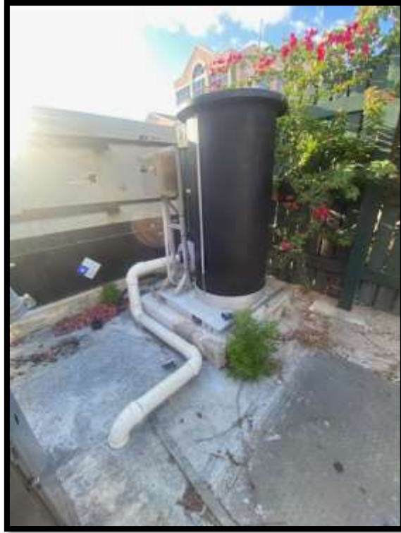
Figure 28. Chlorination station. Source: PlanEHS, 2024.
