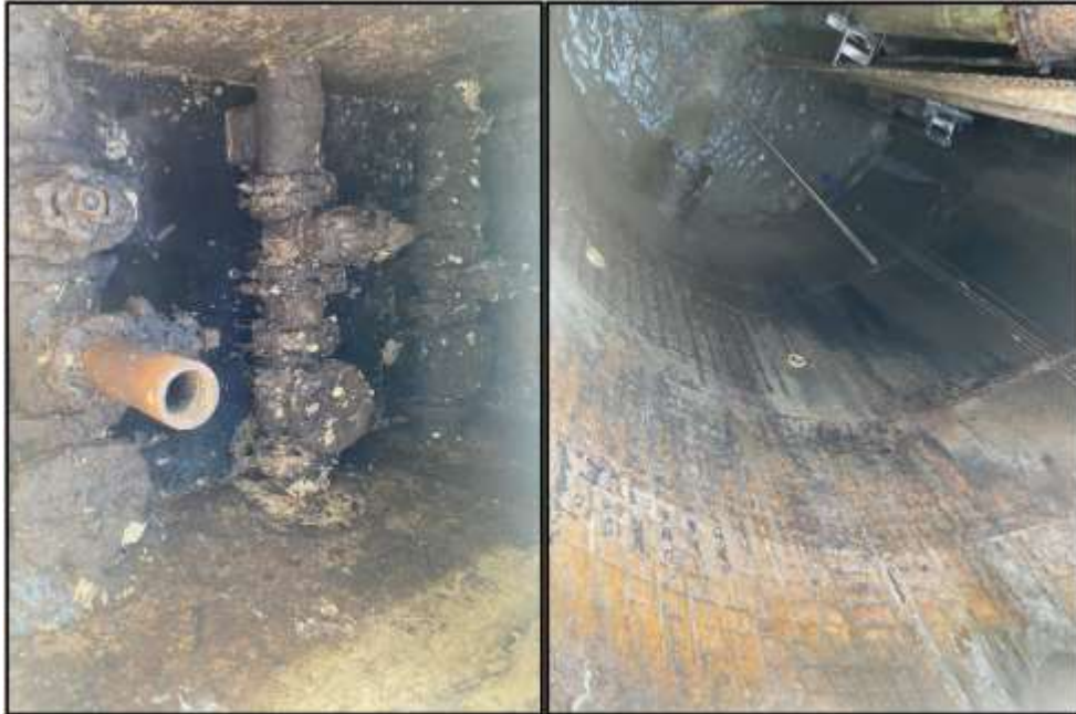
Figure 134. Elizabeth East Lift Station conditions: (a) rusted valves in valve chamber; (b) severe deterioration on well chamber. Source: PlanEHS, 2024.
