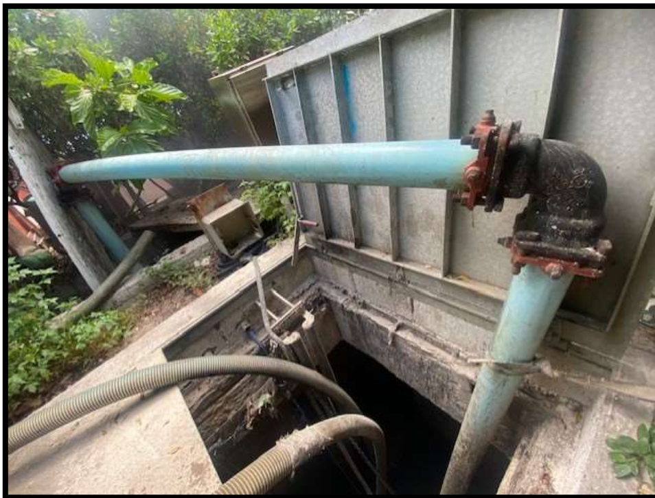
Figure 39. Well chamber and temporary gadget connecting to valve chamber. Source: PlanEHS, 2024.
