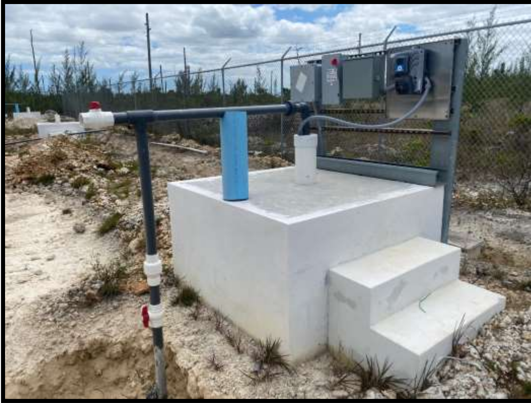
Figure 166. Operational Well. Source: PlanEHS, 2024.
