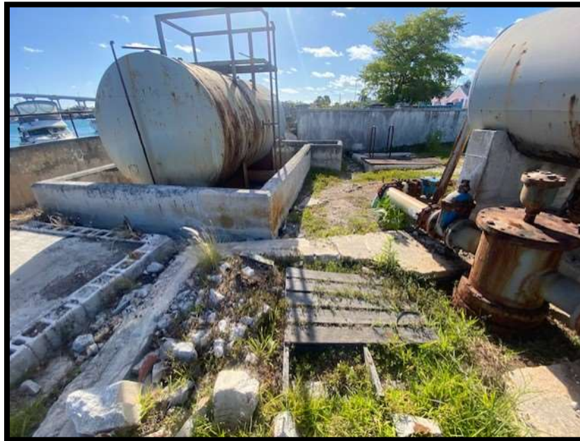
Figure 146. Unused fuel tanks that need to be removed from the premises. Source: PlanEHS, 2024.
