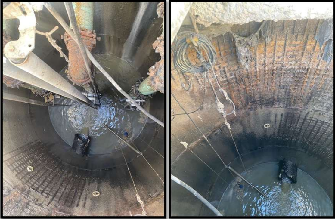
Figure 24. Well Chamber of Elizabeth East LS. Source: PlanEHS, 2024.
