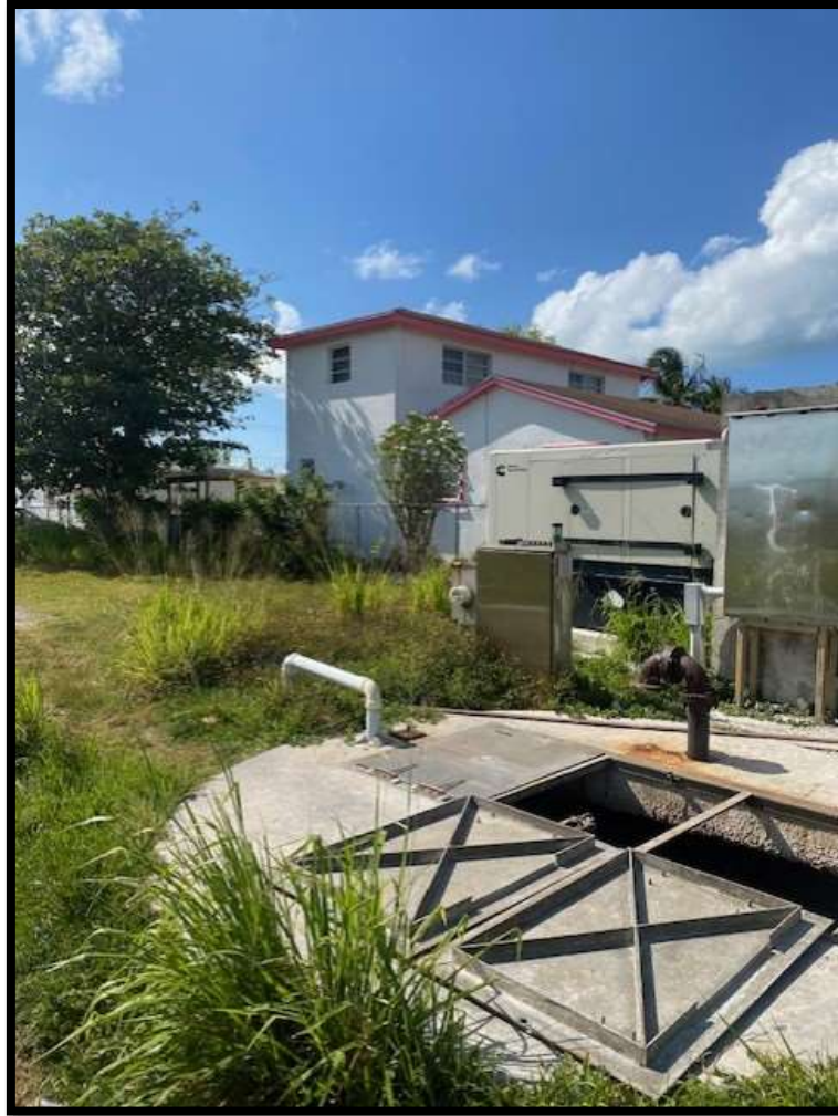
Figure 22. Well Chamber, Pump Control Panel, ventilation, and Power Generator in Elizabeth East LS. Source: PlanEHS, 2024
