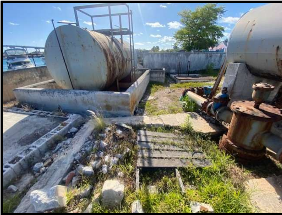
Figure 36. Injection well (right) and unused fuel tank (left) and screening tank (right). Source: PlanEHS, 2024.
