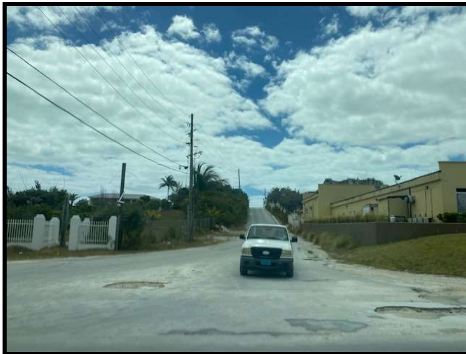
Figure 99. Entrance to Sweetings Tract, Great Abaco Highway and John Sweetings Drive. Source: PlanEHS, 2024.
