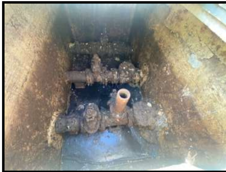
Figure 23. Valve Chamber. Source: PlanEHS, 2024.
