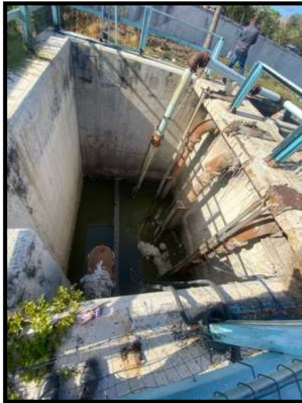
Figure 35. 3 o well chamber and bypass from blue building. Source: PlanEHS, 2024
