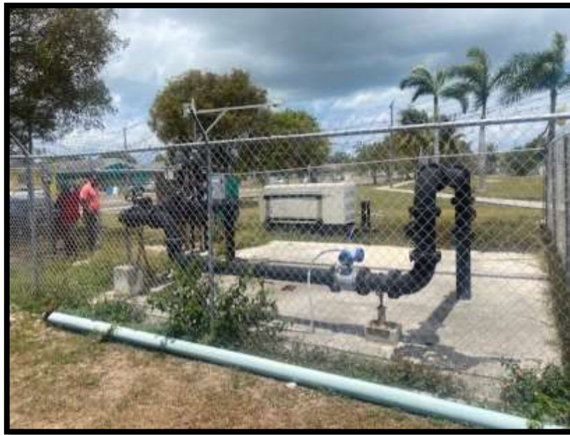
Figure 17. Flamingo C Lift Station. Source: PlanEHS, 2024
