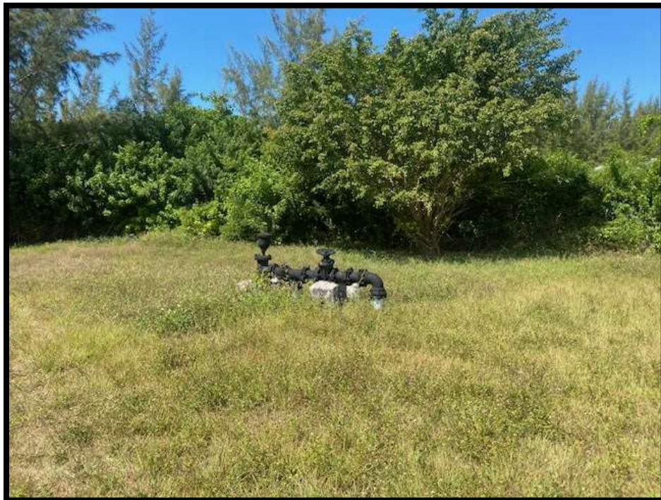
Figure 173. Injection well for treated wastewater. Source: PlanEHS, 2024.
