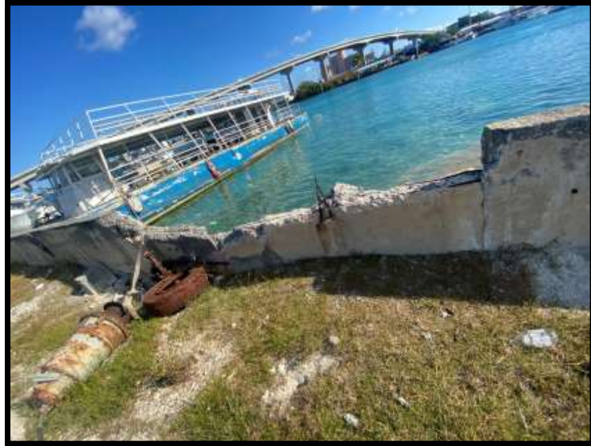
Figure 147. Severe deterioration on seawall and unused equipment. Source: PlanEHS, 2024.
