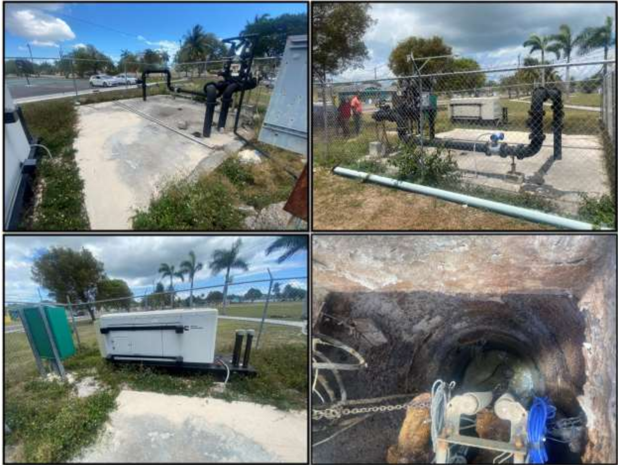
Figure 128. Flamingo C Lift Station: (a) Overground valve system; (b) replaced pipeline; (c) power generator; (d) deteriorated well chamber. Source: PlanEHS, 2024.
