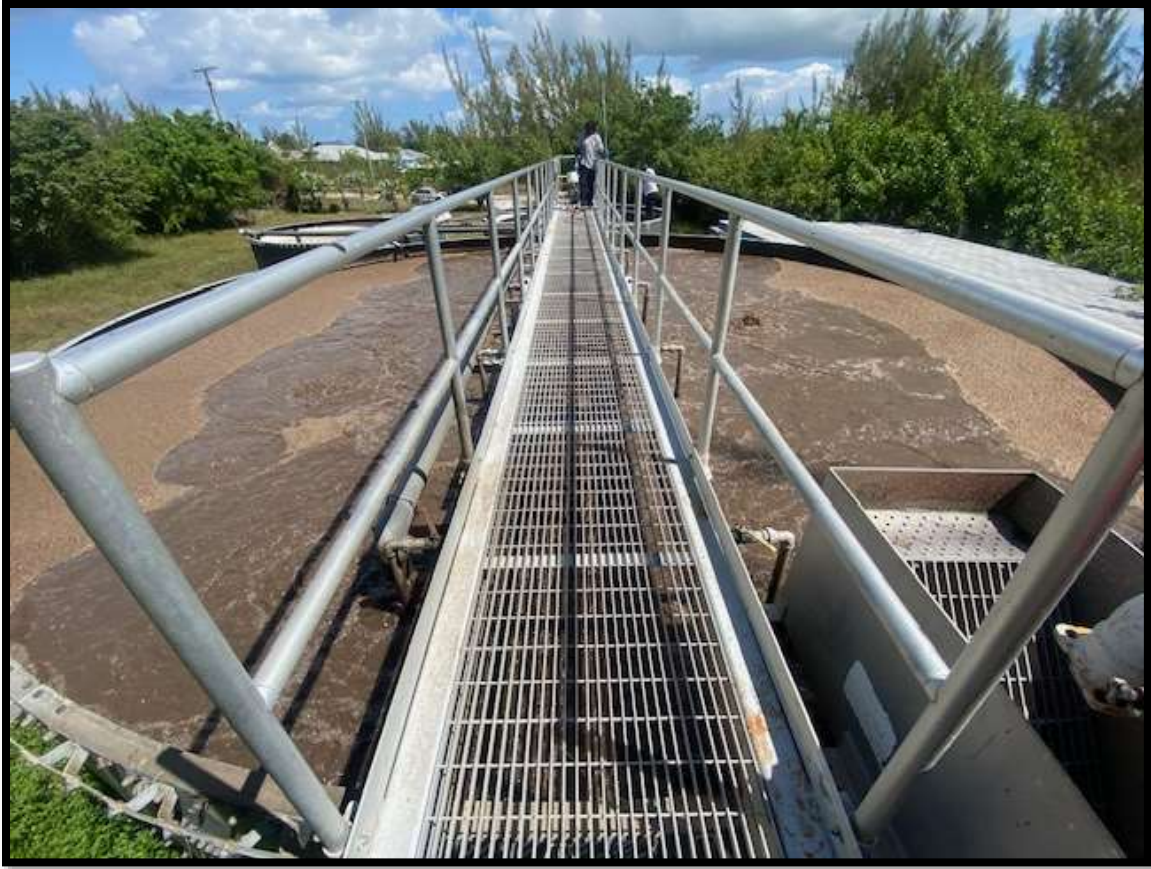
Figure 171. Aeration tank with grid for solid removal (right). Source: PlanEHS, 2024.
