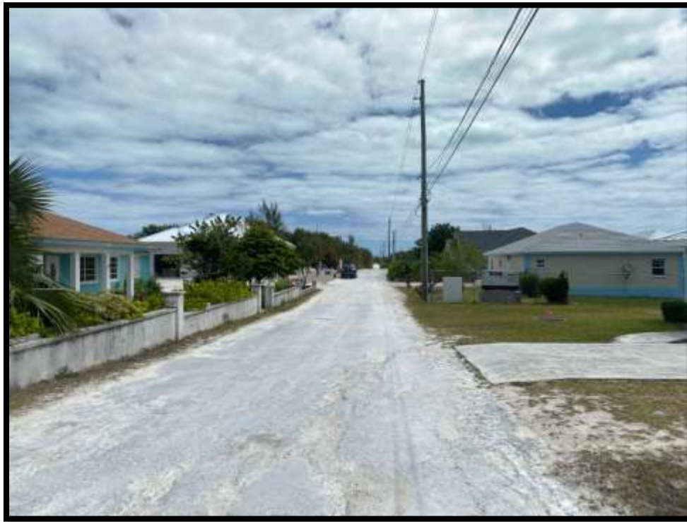
Figure 112. Residential houses and deterioration on paved roads.
