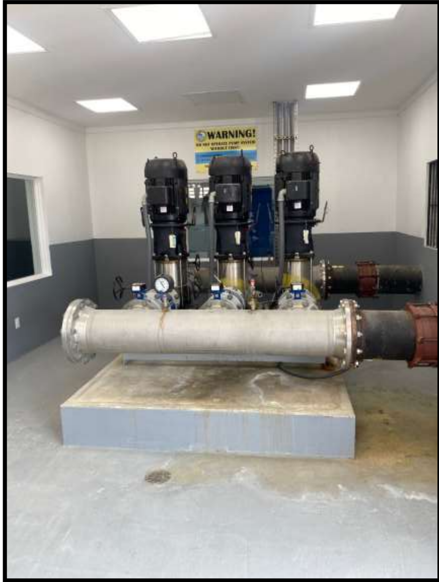
Figure 165. Pumping System at Marsh Harbour Pumping Station. Source: PlanEHS, 2024.
