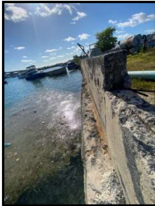
Figure 148. Severe deterioration of seawall and outlet to the sea from the Lift Station. Source: PlanEHS, 2024.
