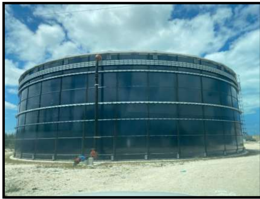
Figure 168. New 1.5 million imperial gallon storage tank. Source: PlanEHS, 2024.
