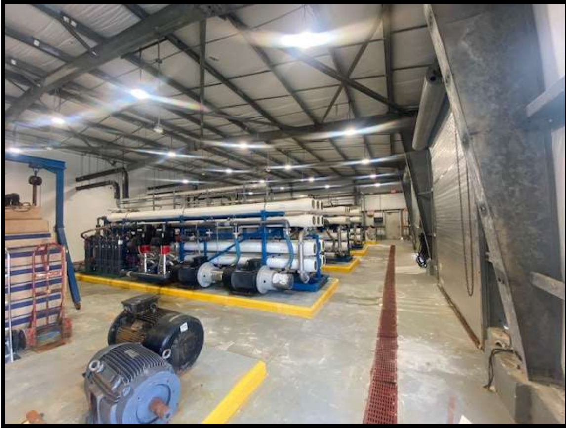
Figure 155. Reverse Osmosis Plant with RO membranes. Source: PlanEHS, 2024.
