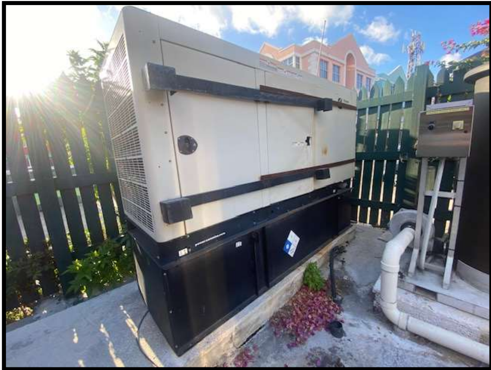
Figure 29. Power Generator. Source: PlanEHS, 2024.
