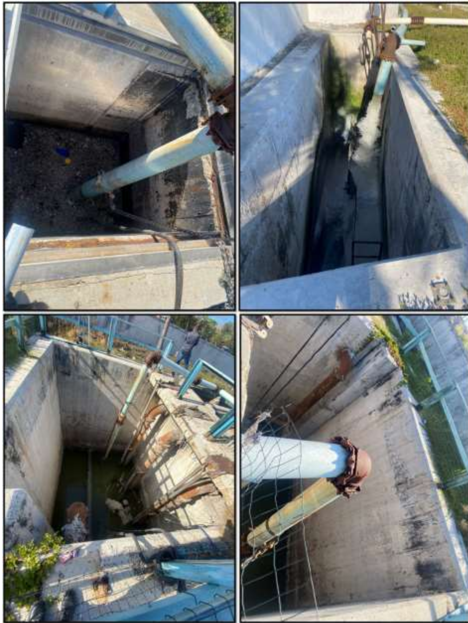
Figure 149. Uncovered well chambers in Malcolm Park Lift Station. Source: PlanEHS, 2024.
