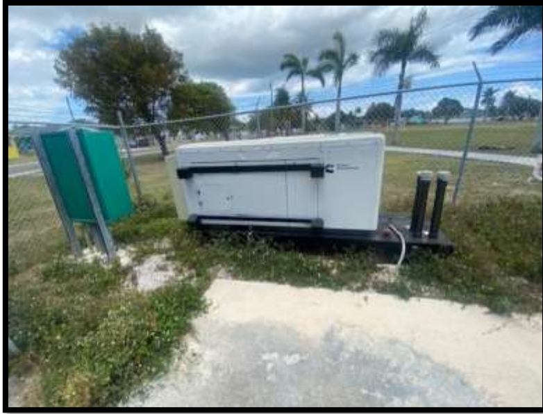
Figure 20. Power Generator. Source: PlanEHS, 2024.
