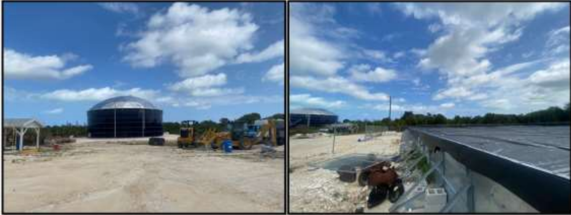
Figure 148. Treated water accumulation tanks: (a) New 1,000,000-gallon tank; (b) Collapsible tank. Source: PlanEHS, 2024.
