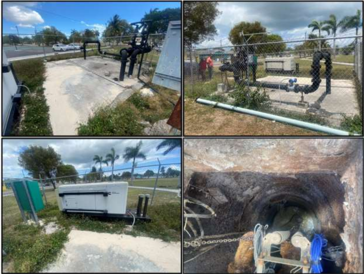
Figure 117. Flamingo C Lift Station: (a) Overground valve system; (b) replaced pipeline; (c) power generator; (d) deteriorated well chamber. Source: PlanEHS, 2024.
