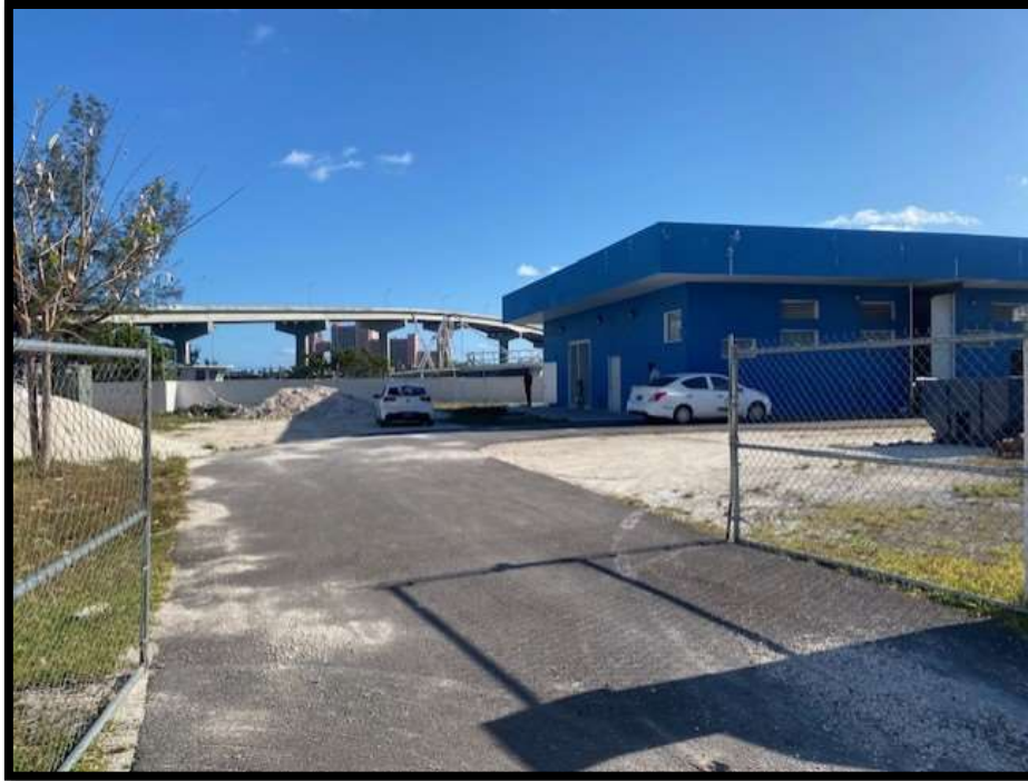
Figure 30. Entrance to Malcom Park Lift Station and nonoperational plant (blue building). Source: PlanEHS, 2024.
