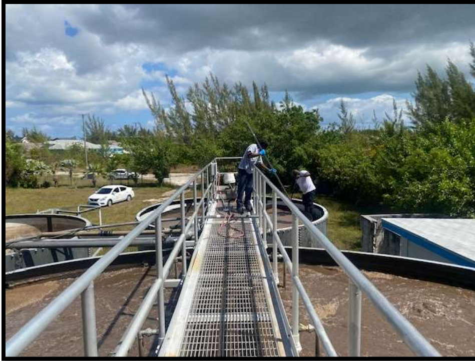
Figure 161. View of Aeration, Clarifier and Digestion Tanks. Source: PlanEHS, 2024.
