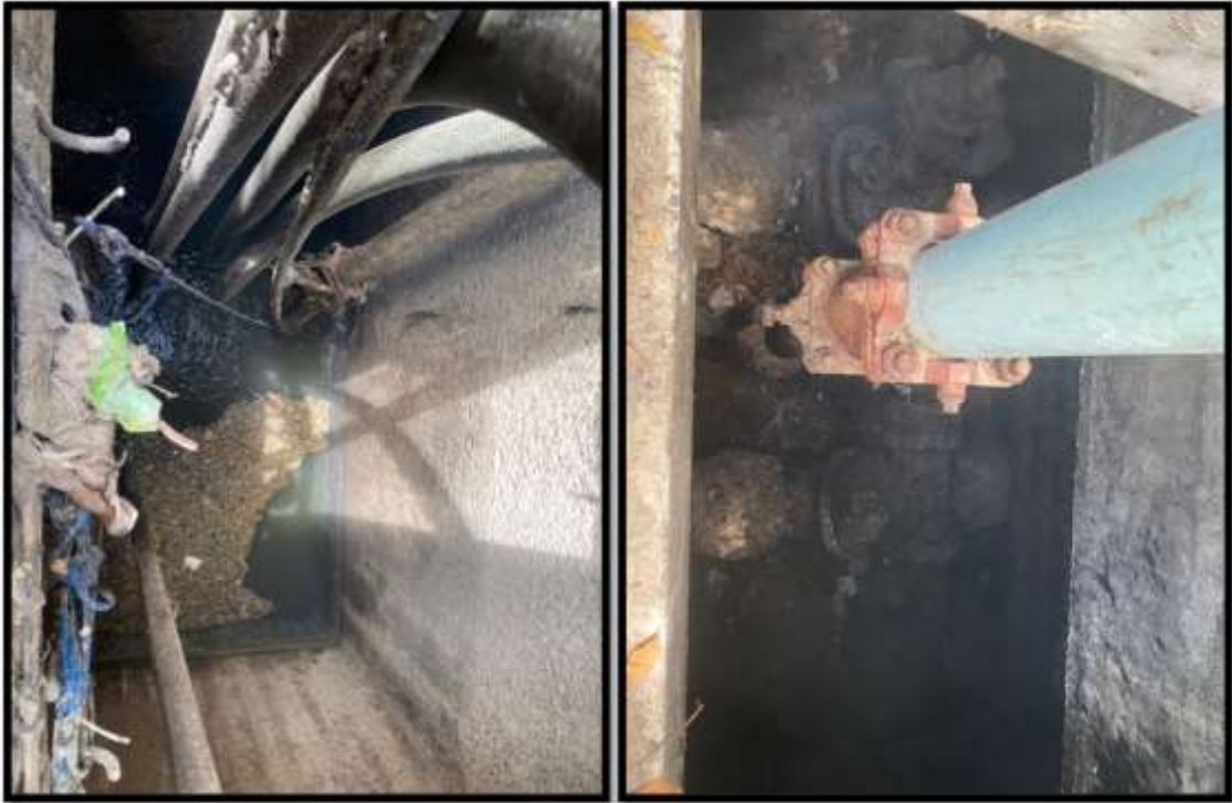
Figure 38. Deterioration on well chamber and valve chamber. Source: PlanEHS, 2024.
