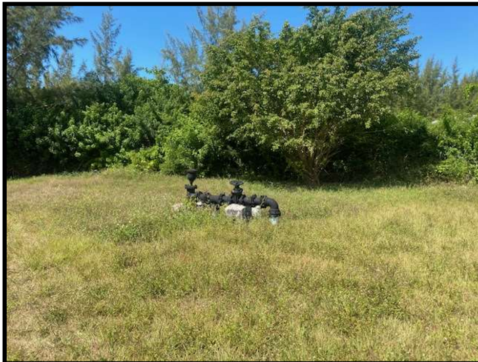
Figure 162. Injection well for treated wastewater. Source: PlanEHS, 2024.
