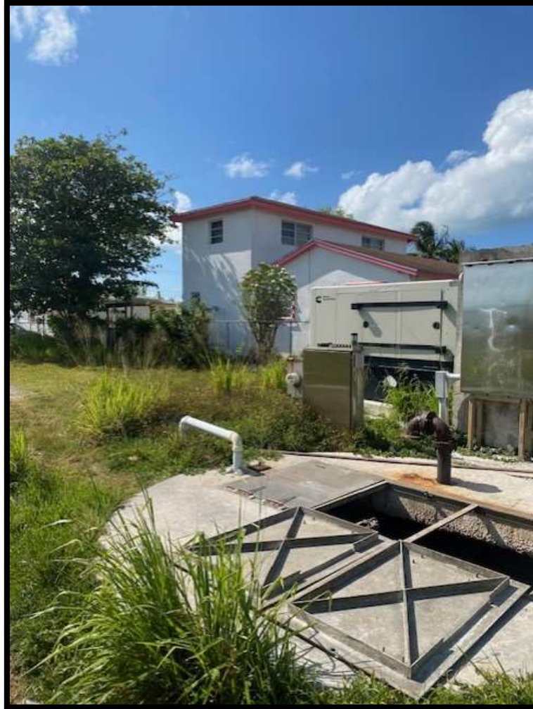
Figure 20. Well Chamber, Pump Control Panel, ventilation, and Power Generator in Elizabeth East LS. Source: PlanEHS, 2024
