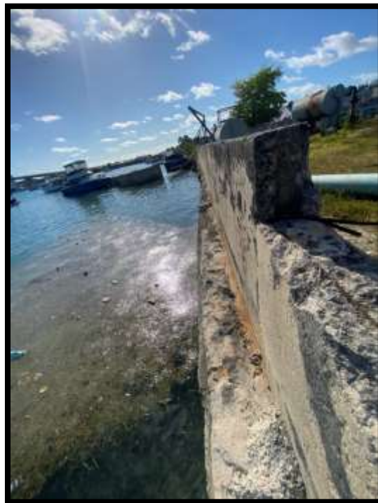
Figure 137. Severe deterioration of seawall and outlet to the sea from the Lift Station. Source: PlanEHS, 2024.
