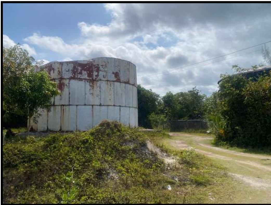
Figure 149. Unused Damaged tank. Source: PlanEHS, 2024.
