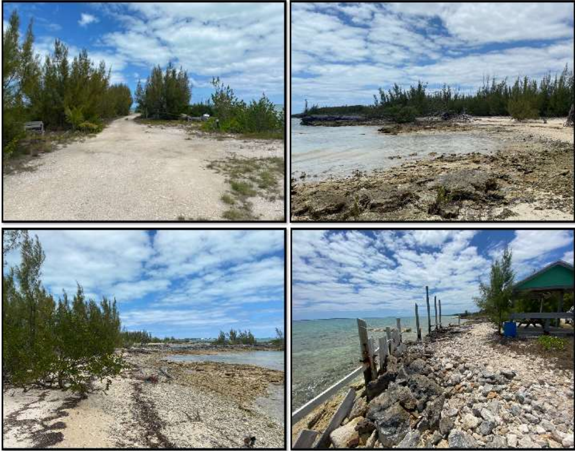
Figure 109. Coastal Area with no seawall and deteriorated wooden balustrade. Source: PlanEHS, 2024.
