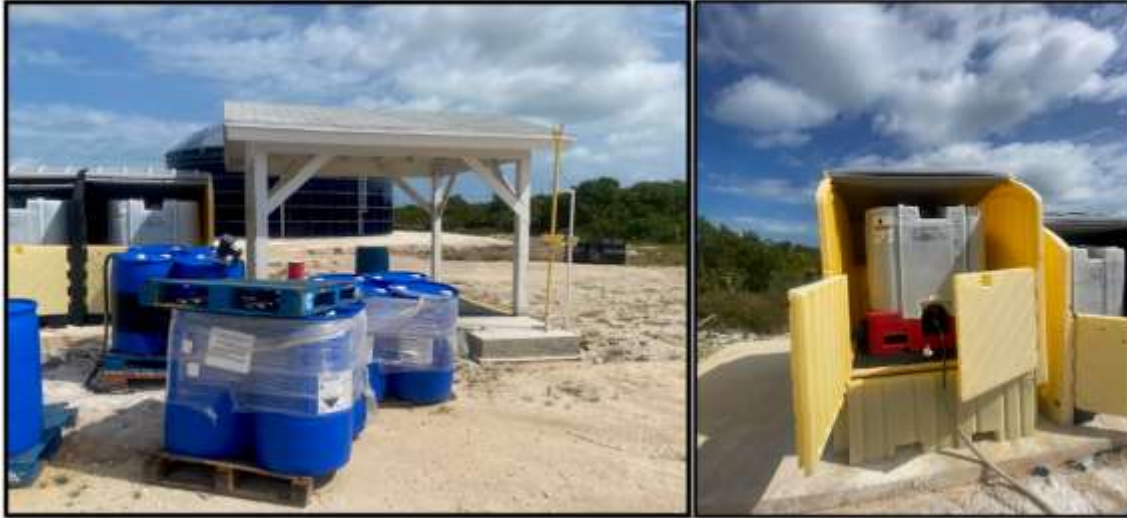
Figure 146. Sulfuric Acid Solution to treat feed water. Source: PlanEHS, 2024.
