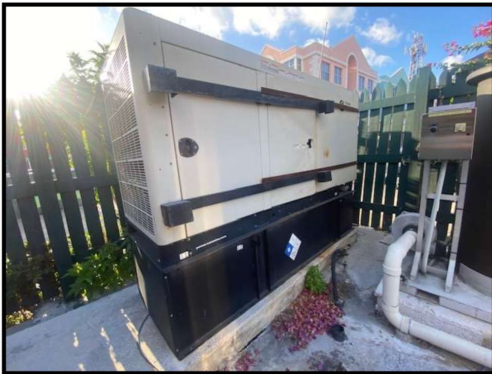
Figure 27. Power Generator. Source: PlanEHS, 2024.
