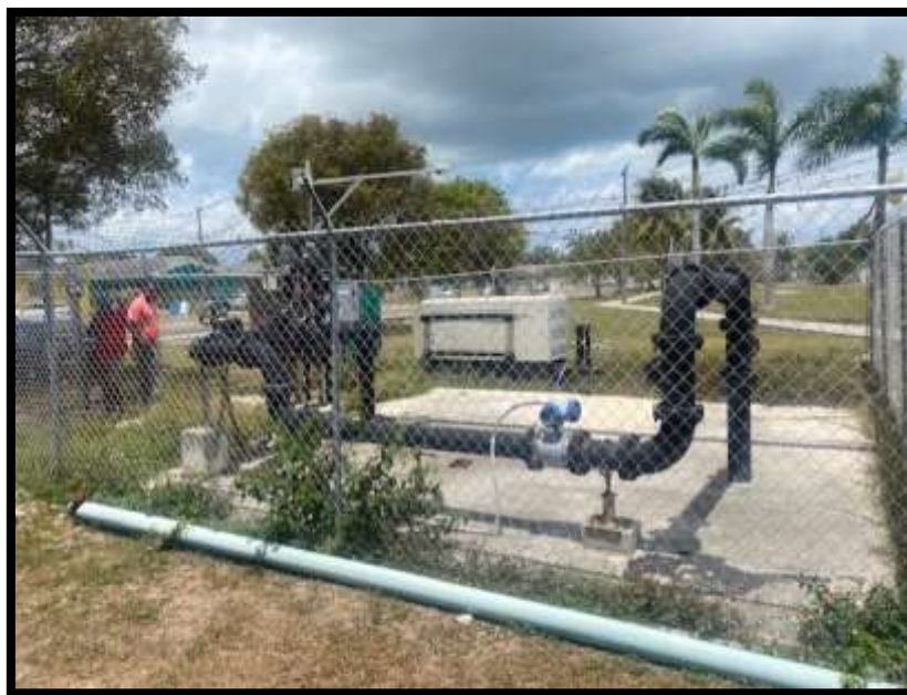
Figure 15. Flamingo C Lift Station. Source: PlanEHS, 2024
