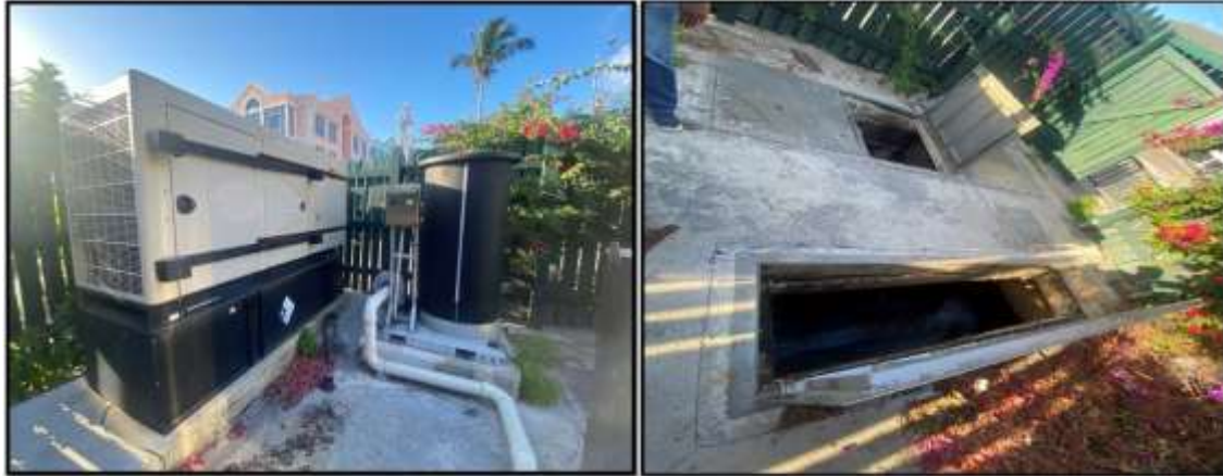
Figure 130. Rawson Square Lift Station: (a) power generator and Chlorination Dosing Machine; (b) well chambers. Source: PlanEHS, 2024.
