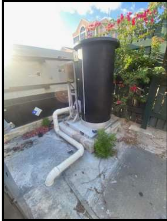
Figure 26. Chlorination station. Source: PlanEHS, 2024.
