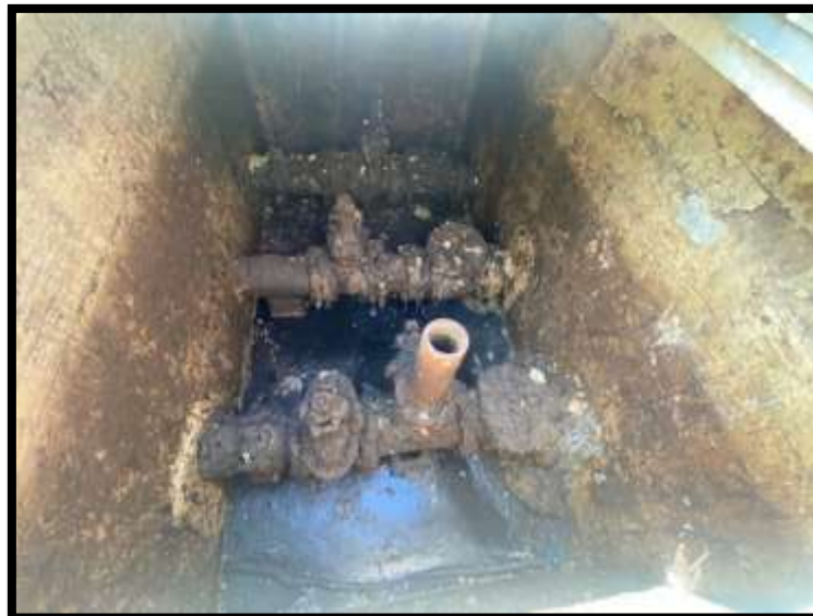
Figure 21. Valve Chamber. Source: PlanEHS, 2024.
