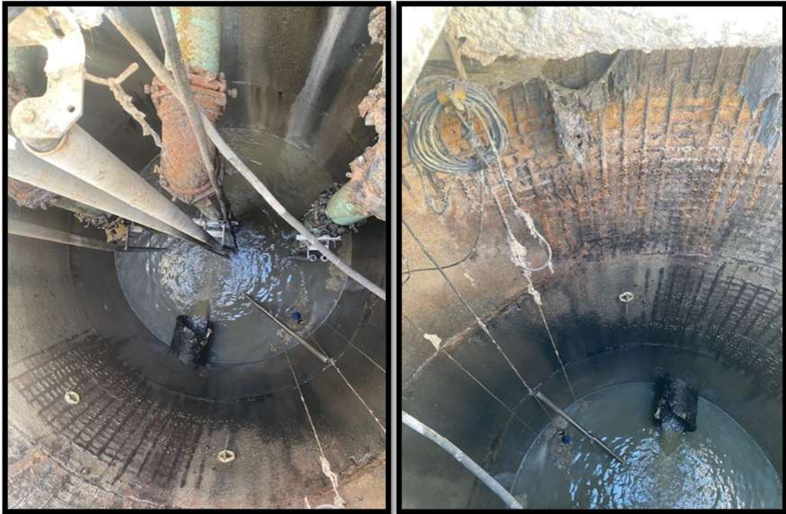
Figure 22. Well Chamber of Elizabeth East LS. Source: PlanEHS, 2024.
