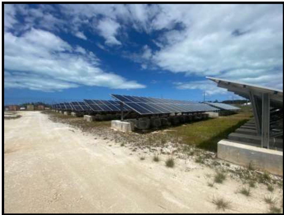
Figure 153. 540 solar panels generating 221KW at Marsh Harbour Pumping Station. Source: PlanEHS, 2024.
