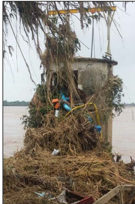
Figure 2.2: Damages to the Main Drinking Water System Intake in Mocuba
