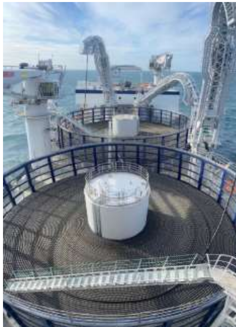
Figure 2-13 – Cable Carousels/turntables. In this case, the vessel is preparing for laying of bundled laying of two power cores for DC (Cigrè).
