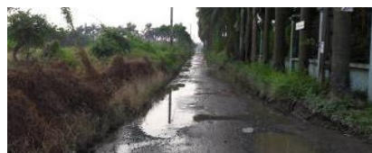
Road in Lane 65, Ngo Xuan Quang Street - adjacent to the construction site of veterinary medicine faculty building - is being degraded - it is also one of the construction items to be funded under this subproject; and will be used as the waste transport route during construction process to the landfill.
