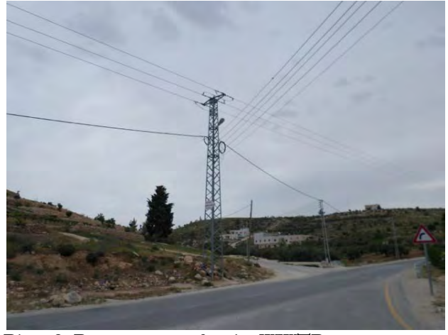
Plate 2: Power source for the WWTP at Hebron – Yatta Road junction
