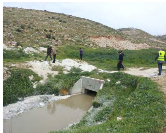
Plate 24: Open wadi channel after the last manhole (proposed wadi access road will not cross-over the wadi)
