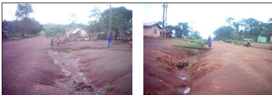
Fig – 4a and 4b: Erosion Problems are common in built-up areas.
