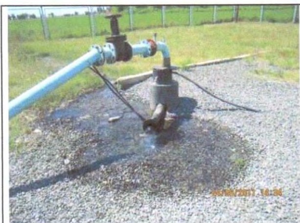
Photo 1: Existing Artisan Bore Well
