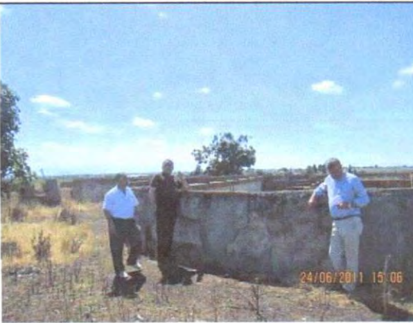
Photo 6: Existing Sewage Treatment Plant (dilapidated & non-functional)
