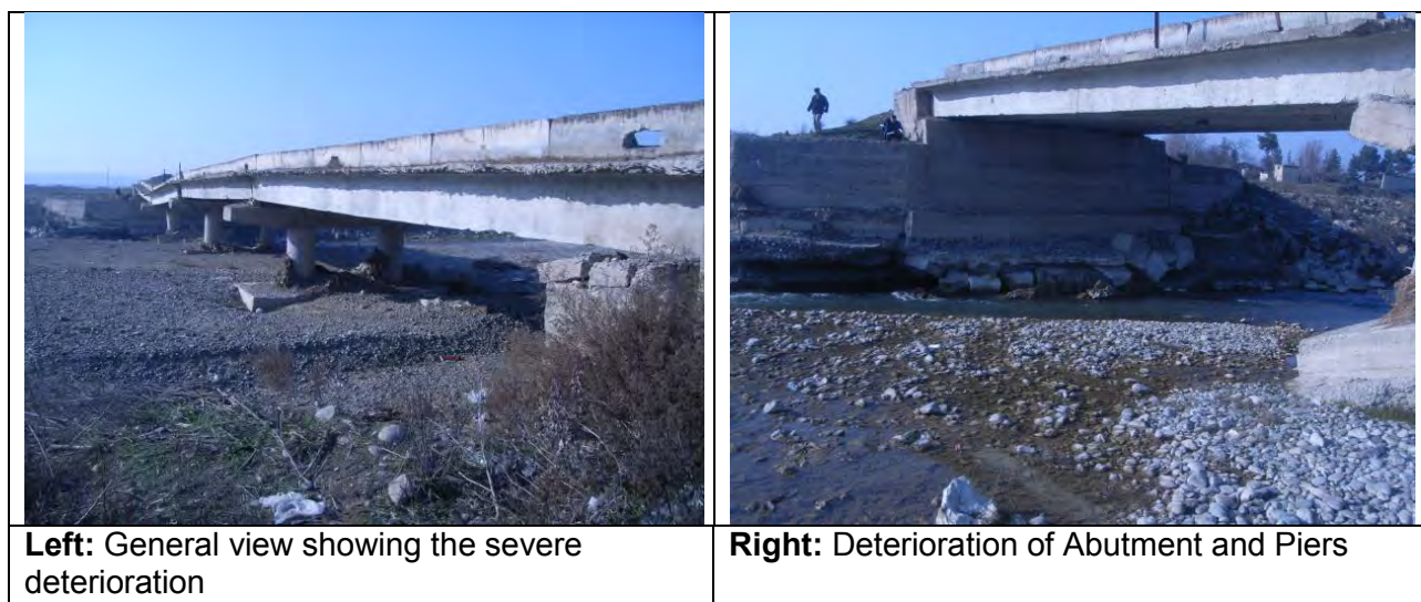
Figure 5: Photographs showing damage of Bridge No. 4
