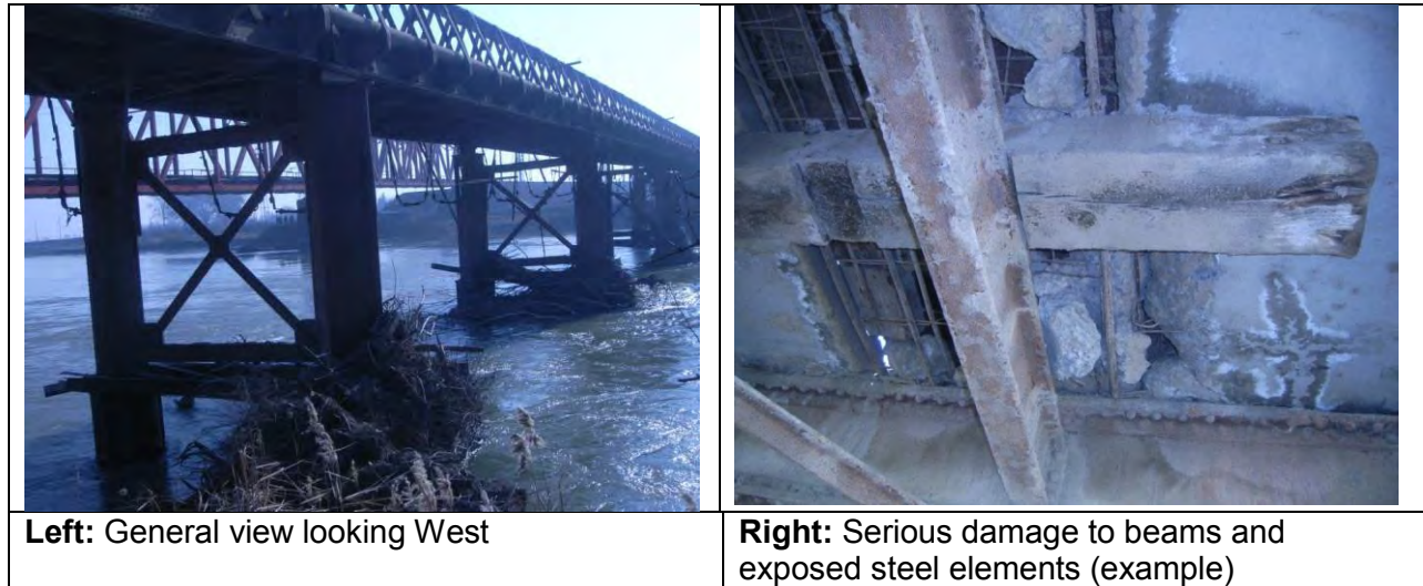
Figure 3: Photographs showing damage of Bridge No. 2
