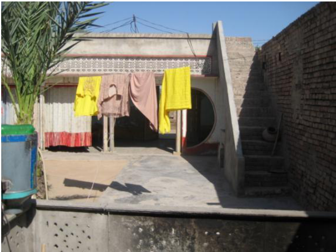
An Affected Structure of Cement and Bricks
