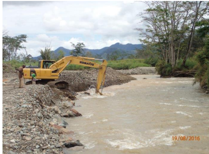
Figure 3 : High-turbidity in Muka River result from material extraction
