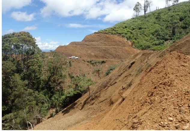
Figure 1: Poor Construction Practices near Km11
