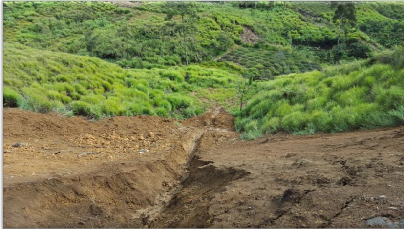
Figure 2 : Dumping of Road side waste at Chainage 51+167
