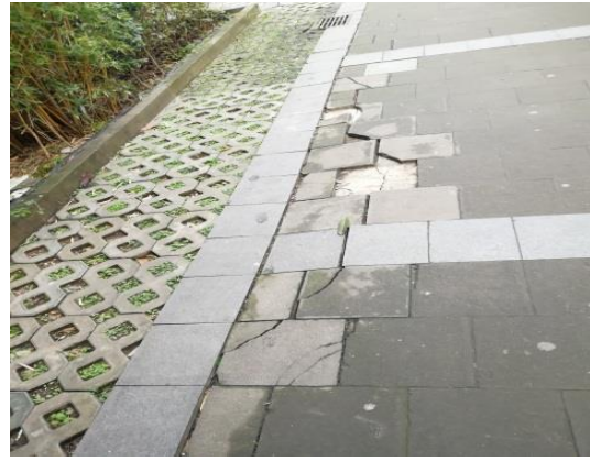
Figure 9-8 Damage of existing footpath
