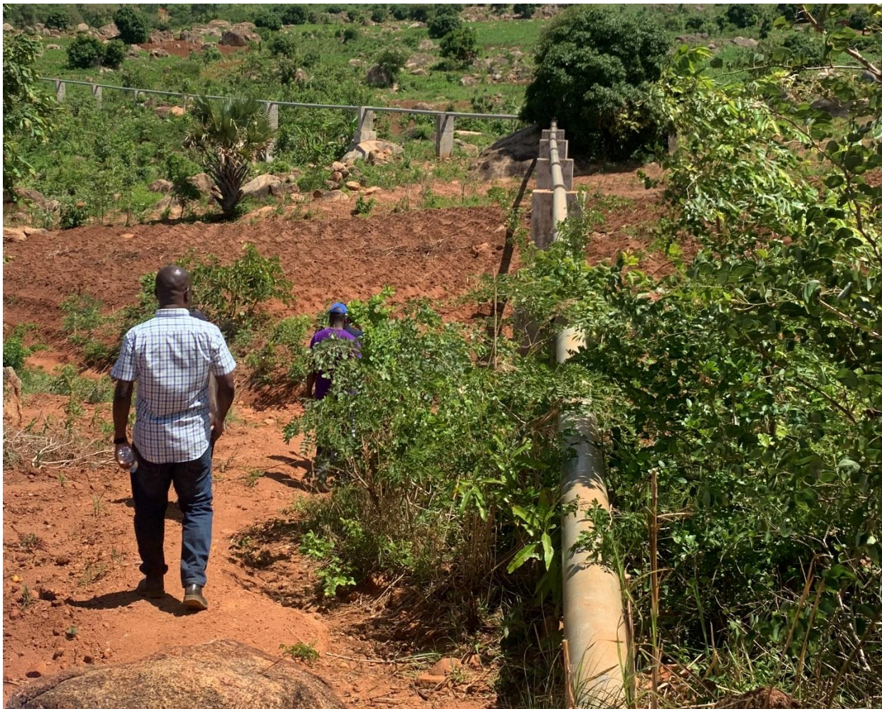
Figure 2.5: Mwaiwathu 200mm IG pipes Conveyance line
