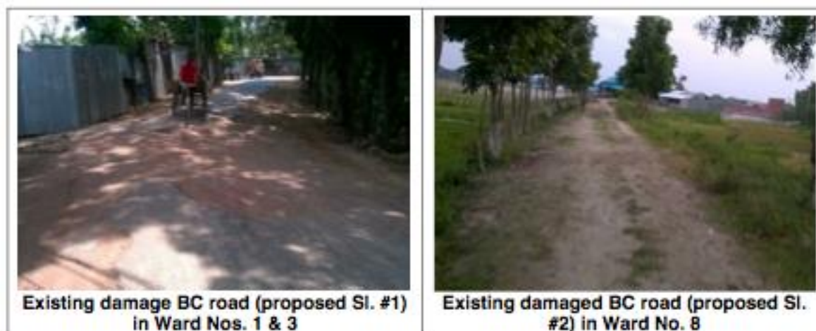
Figure 1: Damaged road of Gopalganj pourashava proposed for development
