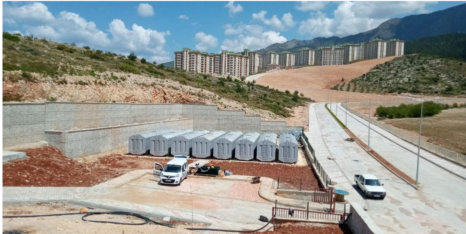
Figure A4.3: Package Wastewater Treatment Plant
