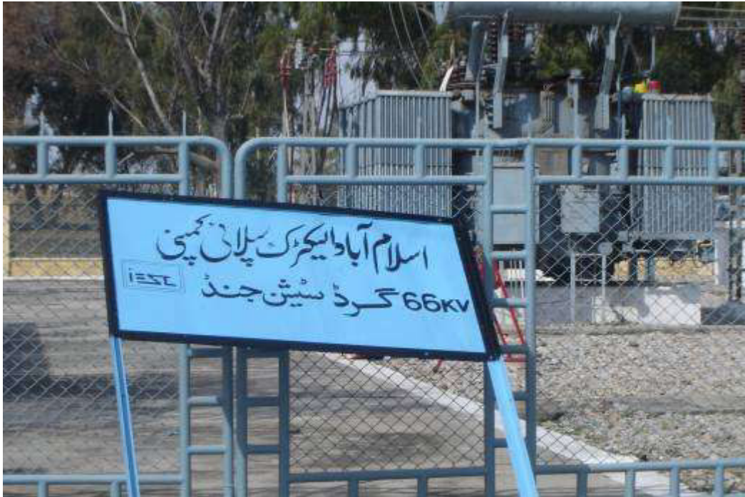
Jand Grid Station site on existing Rawalpindi – Fateh Jang– Kohat Road.
