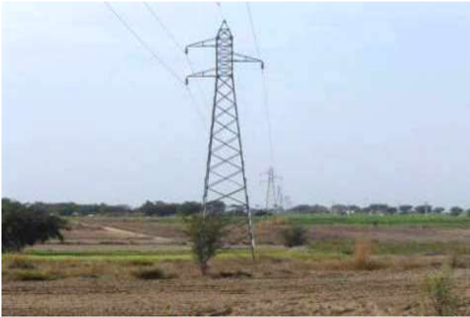
Figure 4.2: Typical Tower 66 KV for cultivated & barren Land.
