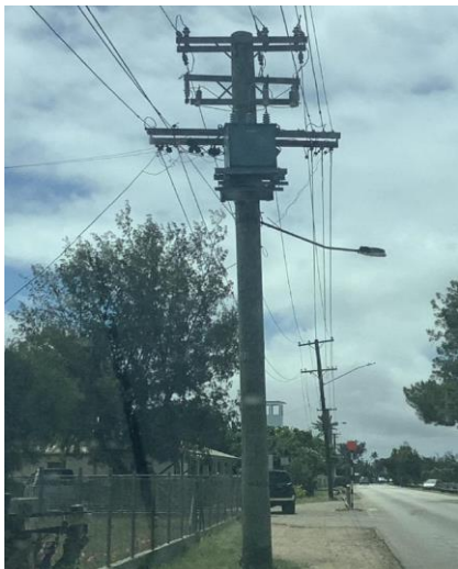
Utility poles and equipment
