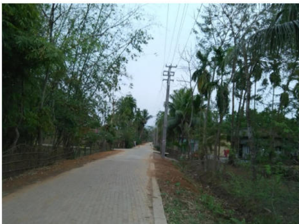
Photo 5: 11kV feeder double line stringing through the village from Singri S/S
