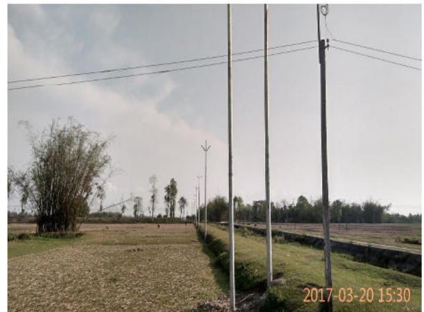
Photo 6: 33kV line tapping from existing 33kV Rowta – Dhekiajuli distribution line for 33/11kV Borsala S/S
