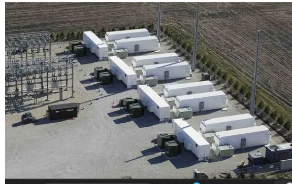
Figure 25: Typical container BESS (external) 9 :
