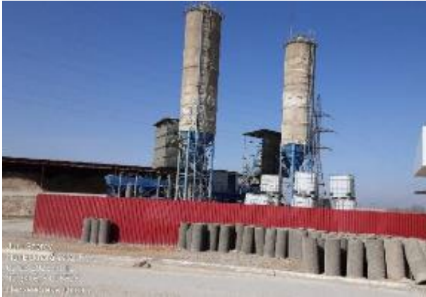
Figure 44: Photo of the batching plant
