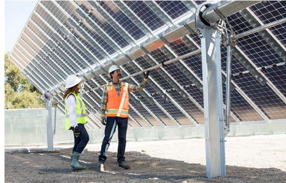
Figure 6: PV tracking system and inverters (Single-axis trackers follow the sun east-to-west on a single point)
