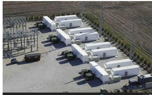
Figure 8: Typical container BESS (external) 1 :
