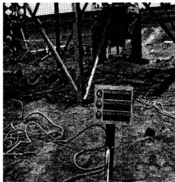
Figure-2: Safety sign placed during erection of tower at Tando Ghulam Ali – Matti TL .
