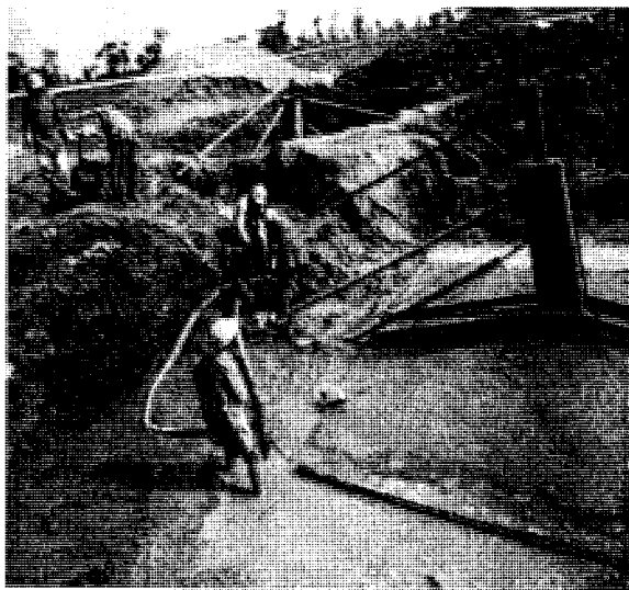
Figure-3: De-watering is in progress during construction of foundation of tower at Haroonabad – Faqeerwali TL
