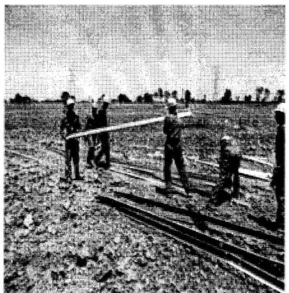
Figure-4: Tower material is being shifted for erection of tower at Nokhar Hafizabad TL ).
