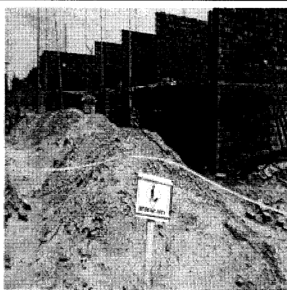
Figure-1: Civil work of control house building in progress at Chonawala GS
