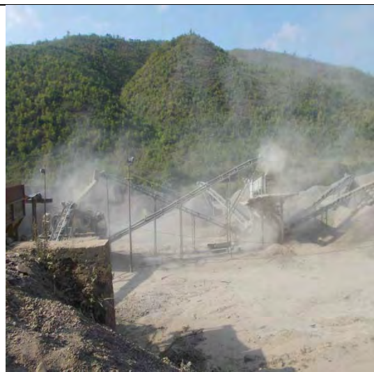
12.Water sprinkling required at crusher area (CW-2)
