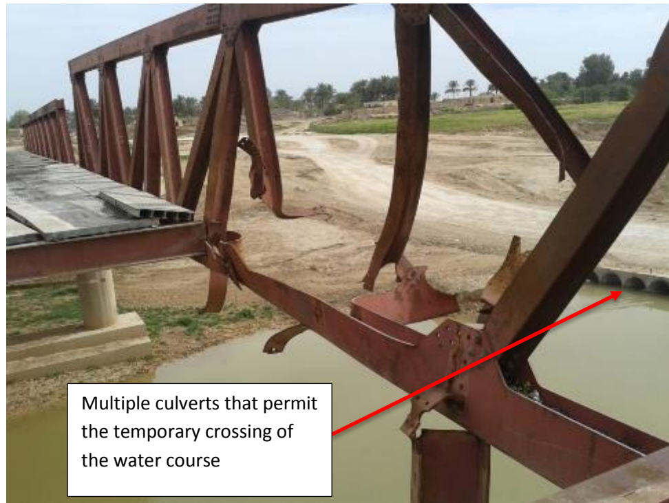
Figure 2: View on the damaged steel bridge and the temporary road currently used
