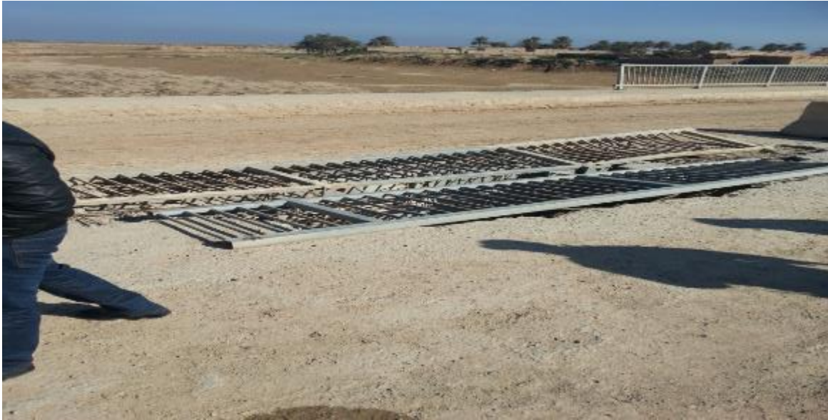
Figure 5: View of the damage on the concrete bridge
