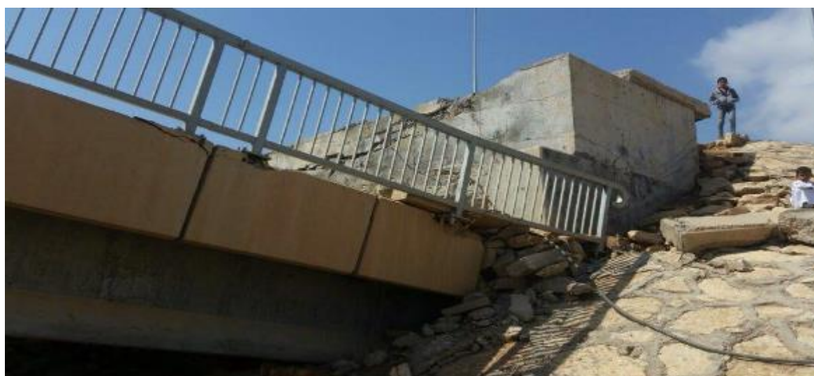
Figure 4: Side view of the damage on the concrete bridge
