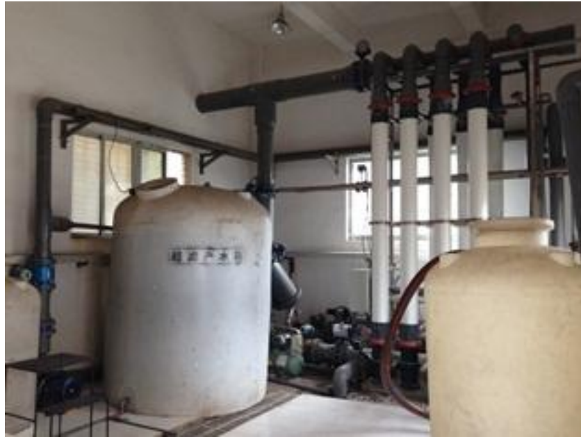
Figure 5-8 Nano-filter unit of leachate treatment in Xishan Incinerator
