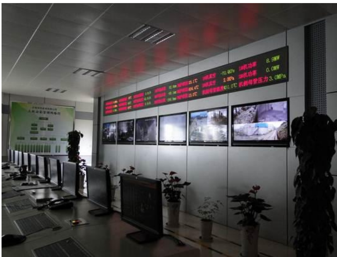
Figure 5-6 Xishan Incineration Plant Central Control Room
