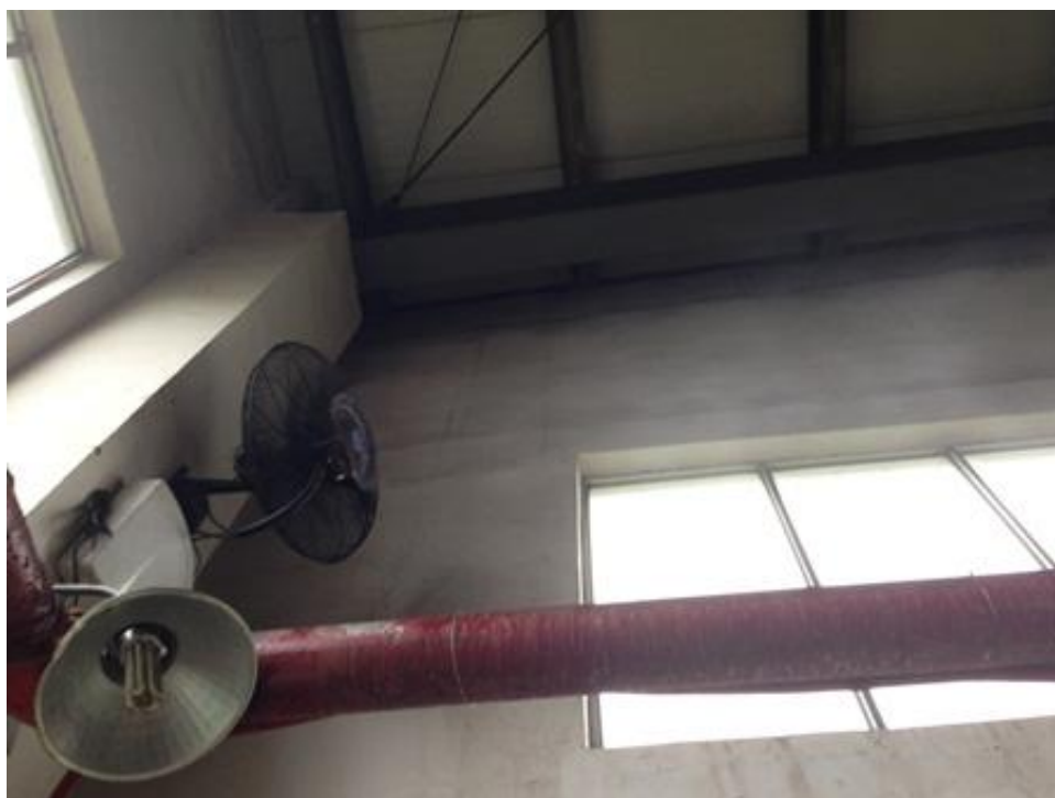
Figure 6-3 Odor Removal at Pretreatment Workshop in Xishan Incinerator
