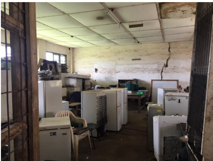
Figure7: Dilapidated Student Workshop at Idi Aba Technical Location
