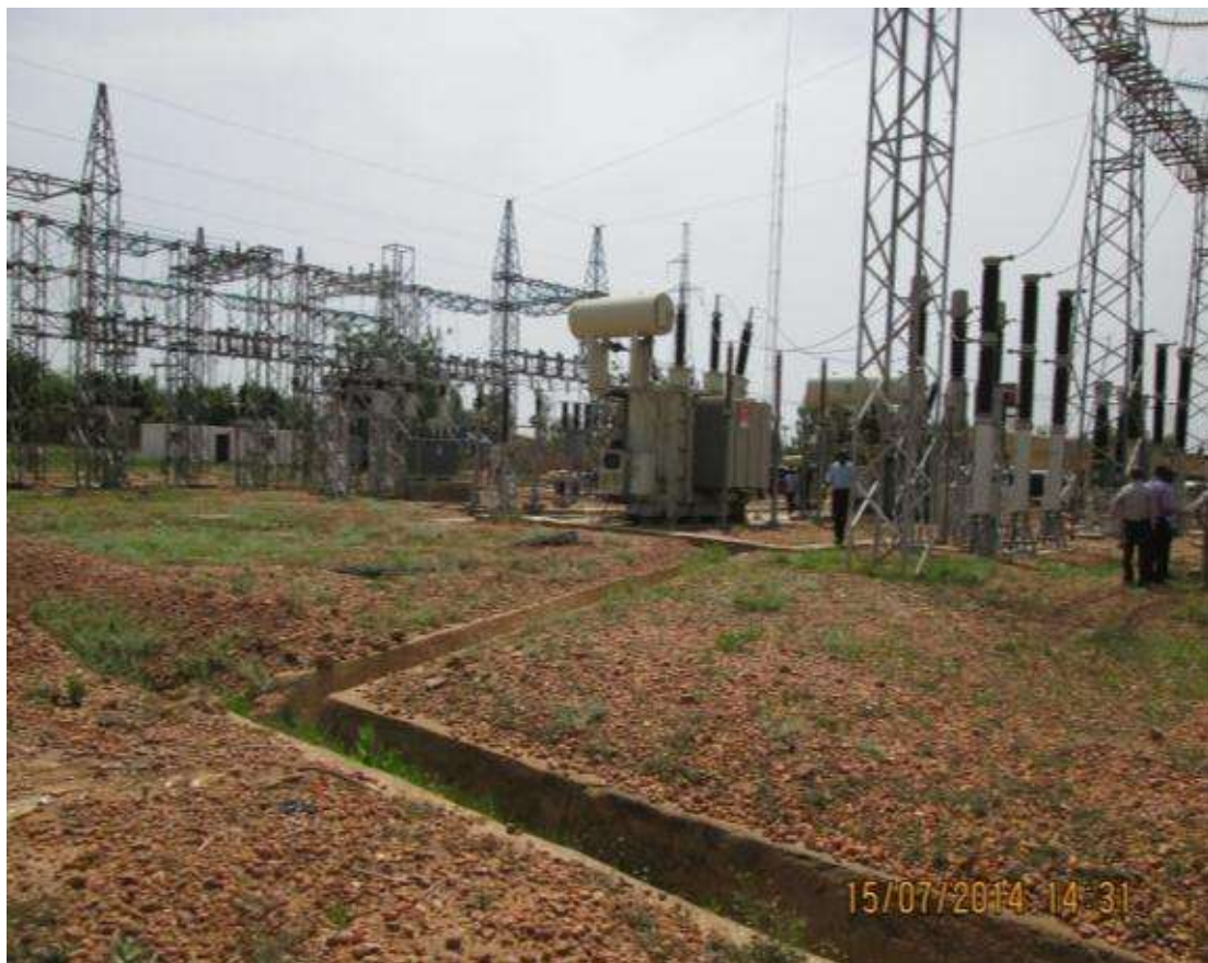
Plate 3.3: A cross-section of existing Kankia Substation
