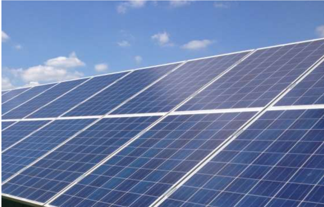
Figure 3.4: Typical Appearance of Polycrystalline Silicon PV Arrays
