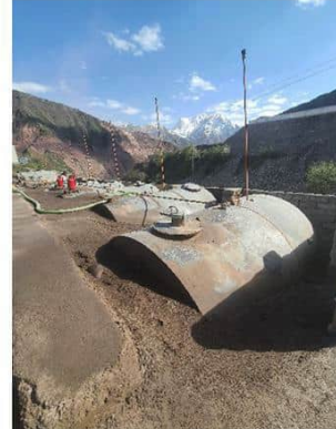
Underground Fuel Storage Tanks
