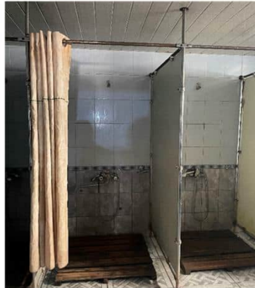
Accommodation Toilets - Inventor
