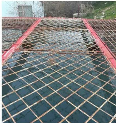
Exposed Drinking Water—Soktmoni Asnsi
