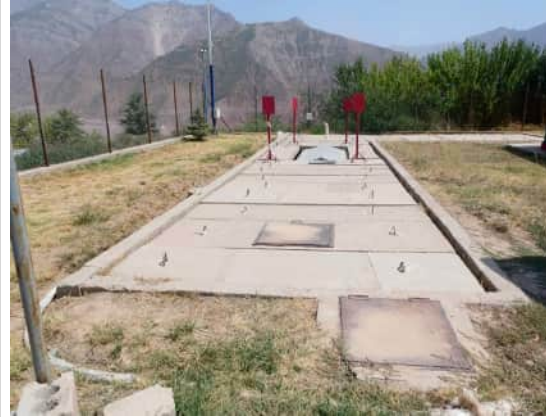
WeBuild Office septic tank
