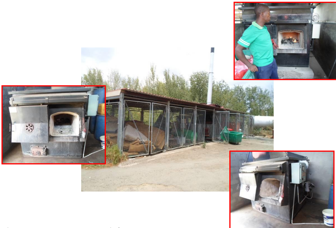
Figure A.3-14 Government Hospital incinerators
