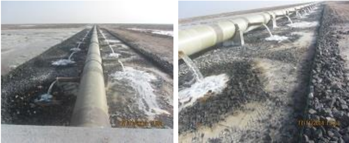
Picture 5.6.5.1. View from the Brine Discharge Line Diffuser Point belonging to Underground Gas Storage Project under leaching studies
