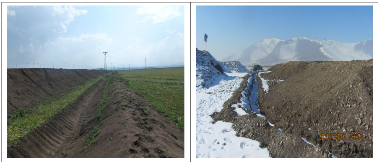
Picture 5.6.6.7. Drainage channels dug in the topsoil storage areas, Photos: B. ERDEM, 2015
