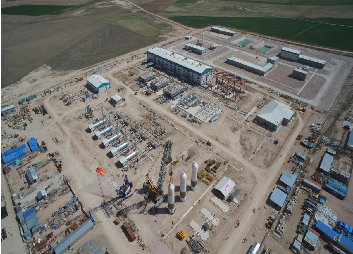
Picture 3.1.1.1. A view of Surface Facilities of Underground Gas Storage Project under Construction
