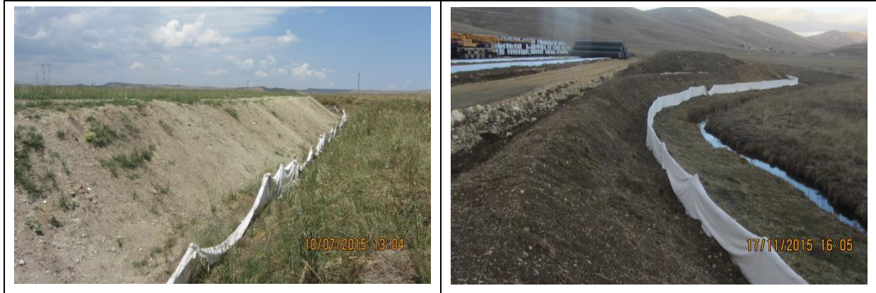
Picture 5.6.6.11. Silt fence applications in topsoil storage areas for the purpose of protection, Photos: B. ERDEM, 2015
